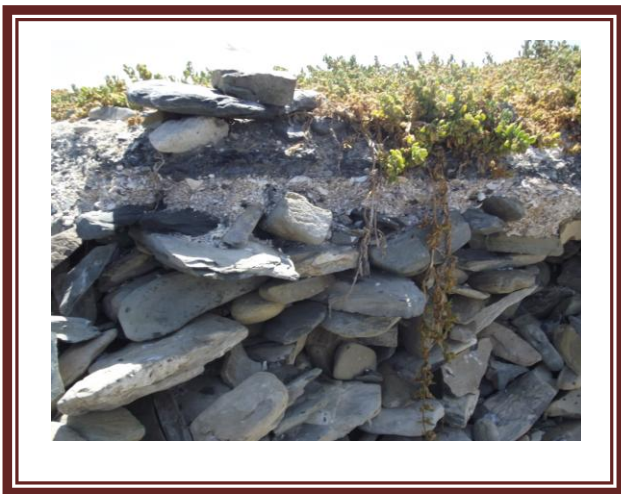
Fig.4. Vegetation on wall
