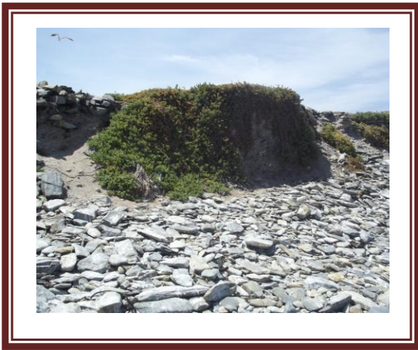
Fig.2. Vegetation over wall
