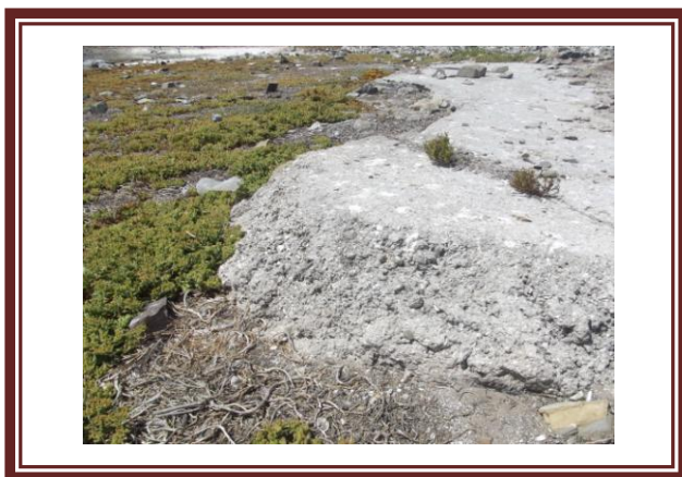
Figures 9 to 11. Showing exposed parts of concrete slab
