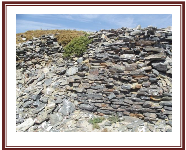
Fig.5. Vegetation on wall
