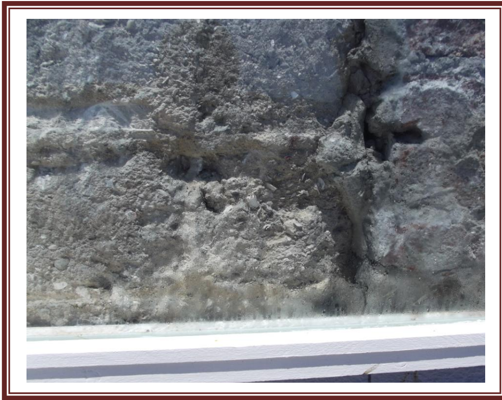
Fig 3 and 4. Showing moisture build up.
