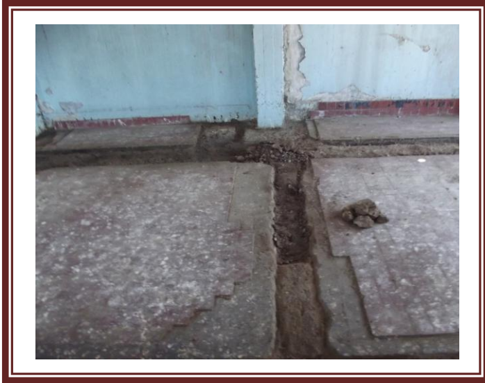
Fig.23. Showing skirting outline with missing tiles.
