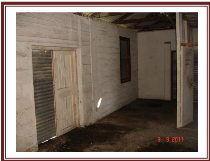
Fig.38. Interior of door boarded up
