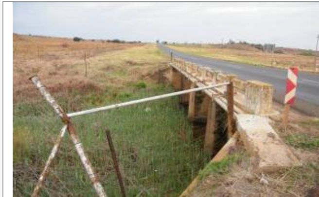
Picture showing the existing Keerom Spruit Bridge taken when looking North. Note the existing bridge infrastructure
