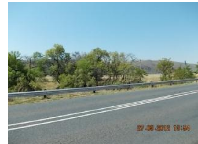
Picture showing culvert 7 over the Kranspoort Spruit Tributary. This picture was taken looking Northeast.
