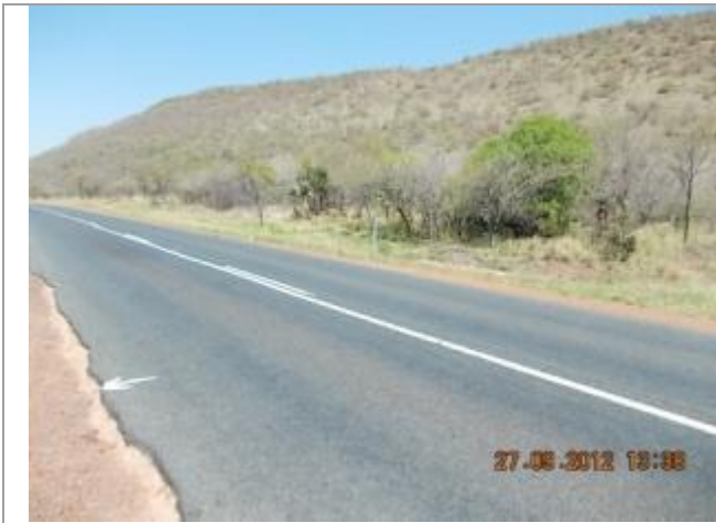
Picture depicting the existing N11 road between Middelburg and Loskop Dam. This picture shows culvert 6 over the Kranspoort Spruit Tributary looking Southeast.
