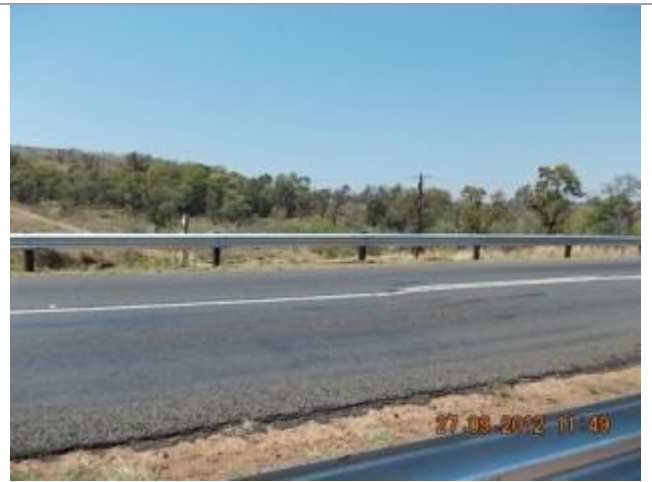
Picture depicting the existing N11 road between Middelburg and Loskop Dam. This picture shows culvert 2 over the Klip River Tributary looking East.
