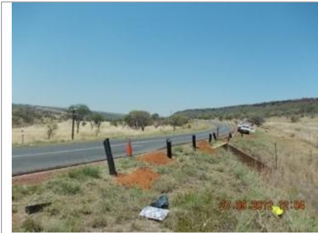
Picture depicting the existing N11 road between Middelburg and Loskop Dam. This picture shows culvert 3 over the Klip River Tributary looking Southeast.
