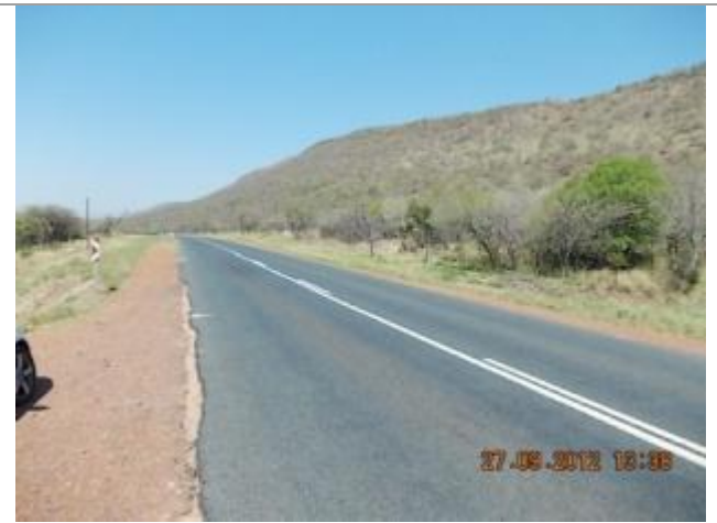
Picture depicting the existing N11 road between Middelburg and Loskop Dam. This picture shows culvert 6 over the Kranspoort Spruit Tributary looking East.
