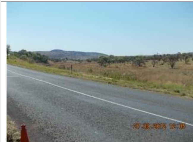
Picture showing culvert 3 across Klip River Tributary. This picture was taken looking Northeast.
