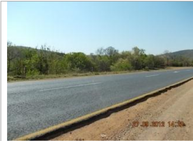
Picture depicting the existing N11 road between Middelburg and the Olifants River Bridge. This picture shows culvert 8 over the Olifants River Tributary looking Northwest.
