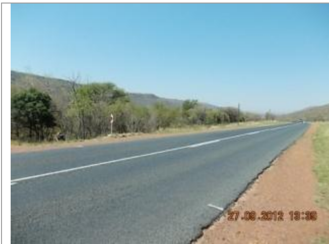
Picture showing the existing culvert 6 across Kranspoort Spruit Tributary. This picture was taken looking Northeast.
