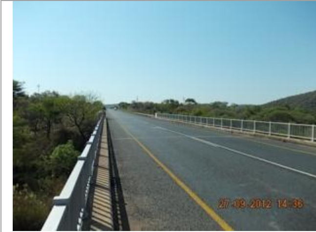
Picture showing the existing bridge 3611 over the Olifants River. This picture was taken looking North.
