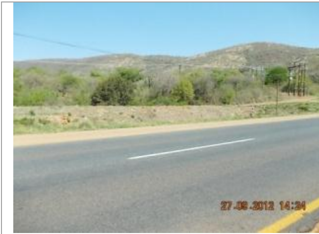
Picture depicting the existing N11 road between Middelburg and the Olifants River Bridge. This picture shows culvert 8 over the Olifants River Tributary looking Southeast.
