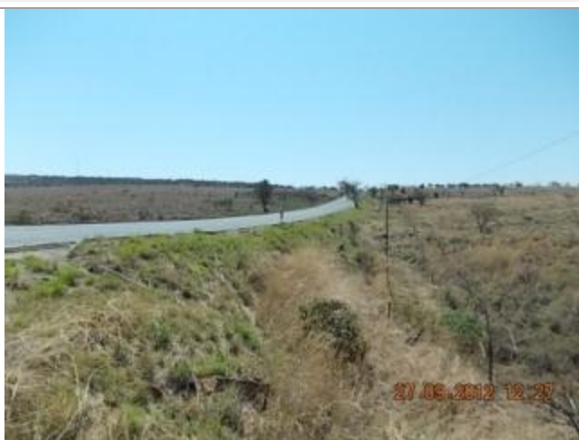
Picture depicting the existing N11 road between Middelburg and Loskop Dam. This picture shows culvert 4 over the Klip River Tributary looking Northwest.
