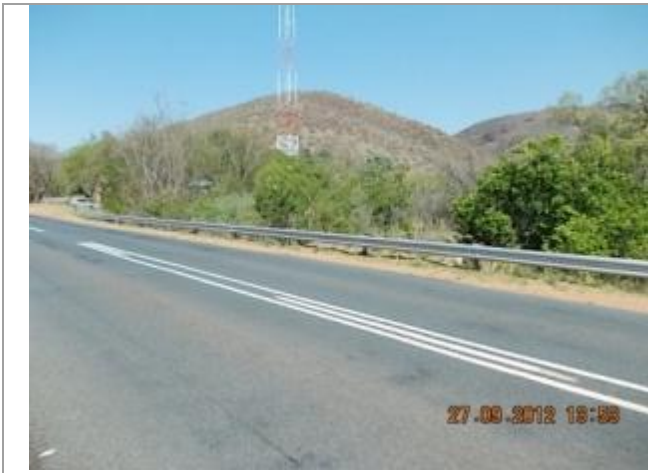
Picture depicting the existing N11 road between Middelburg and Loskop Dam. This picture shows culvert 7 over the Kranspoort Spruit Tributary looking Southeast.
