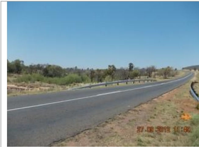
Picture depicting the existing N11 road between Middelburg and Loskop Dam. This picture shows culvert 2 over the Klip River Tributary looking Southeast.
