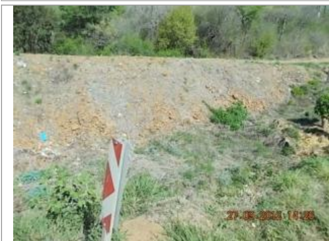
Current wall next to the N11 across the tributary blocking the watercourse.
