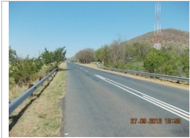
Picture depicting the existing N11 road between Middelburg and Loskop Dam. This picture shows culvert 7 over the Kranspoort Spruit Tributary looking East.
