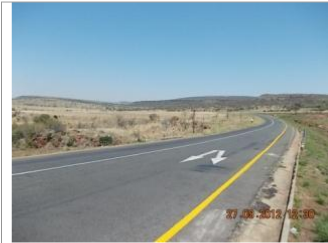
Picture depicting the existing N11 road between Middelburg and Loskop Dam. This picture shows culvert 4 over the Klip River Tributary looking Southeast.
