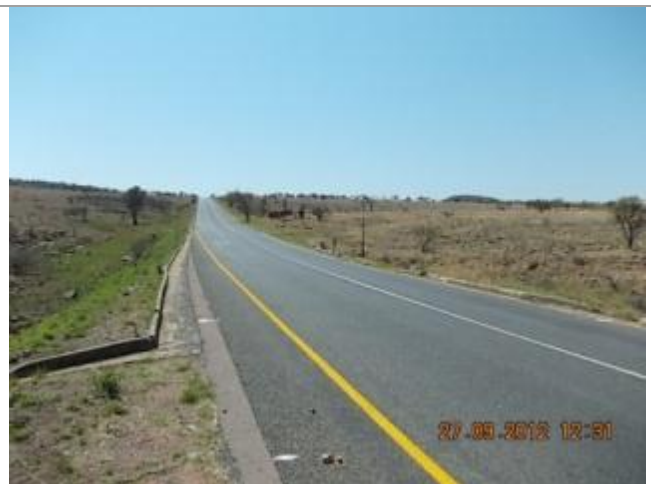
Picture showing culvert 4 across Klip River Tributary. Picture showing the Klip River Tributary looking North.
