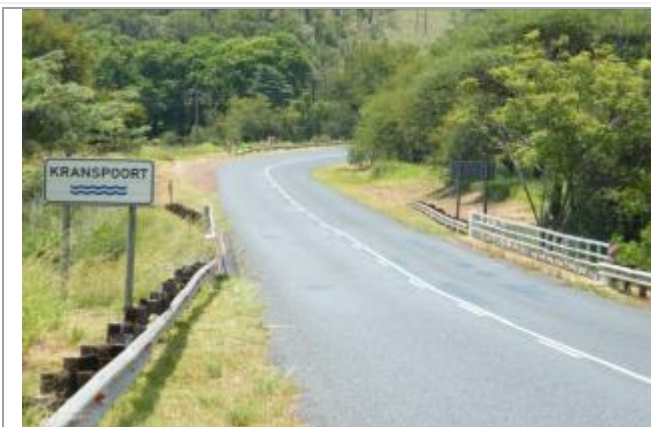
Picture showing the existing bridge across Kranspoort River. This picture was taken looking North
