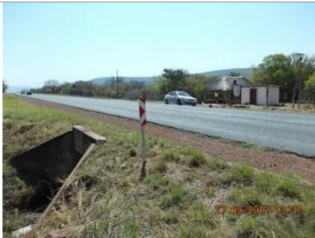
Picture depicting the existing N11 road between Middelburg and Loskop Dam. This picture shows culvert 6 over the Kranspoort Spruit Tributary looking Northwest.
