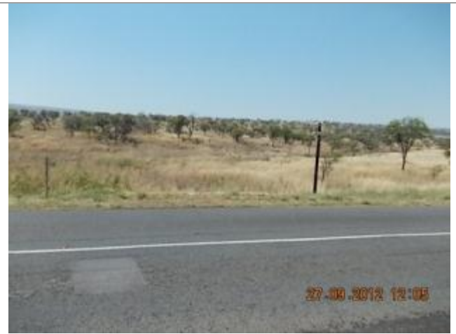
Picture depicting the existing N11 road between Middelburg and Loskop Dam. This picture shows culvert 3 over the Klip River Tributary looking East.
