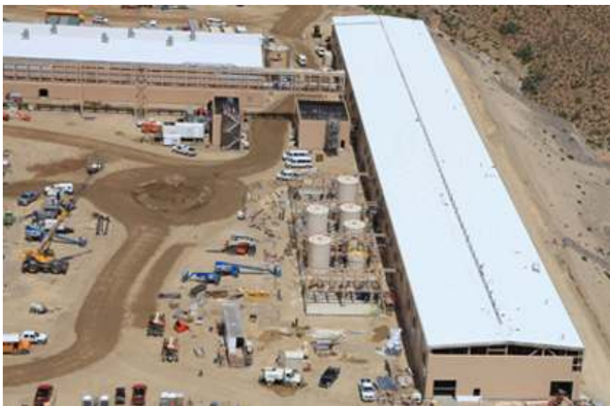
Figure 2: Picture of a typical Rare Earth Separation Plant
