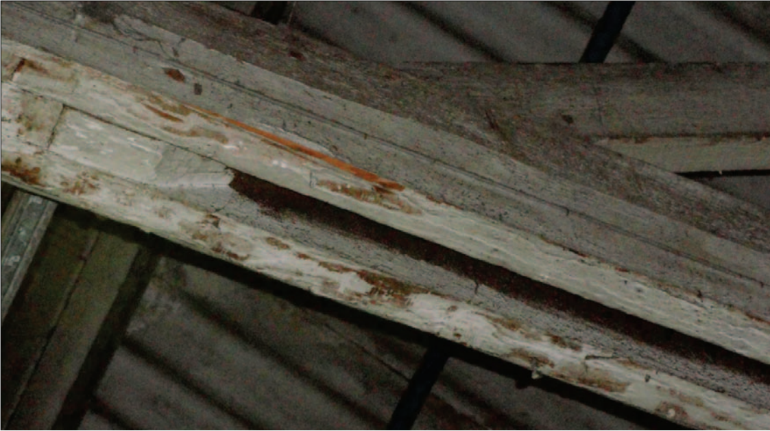
zone 03 | trusses showing borer holes
