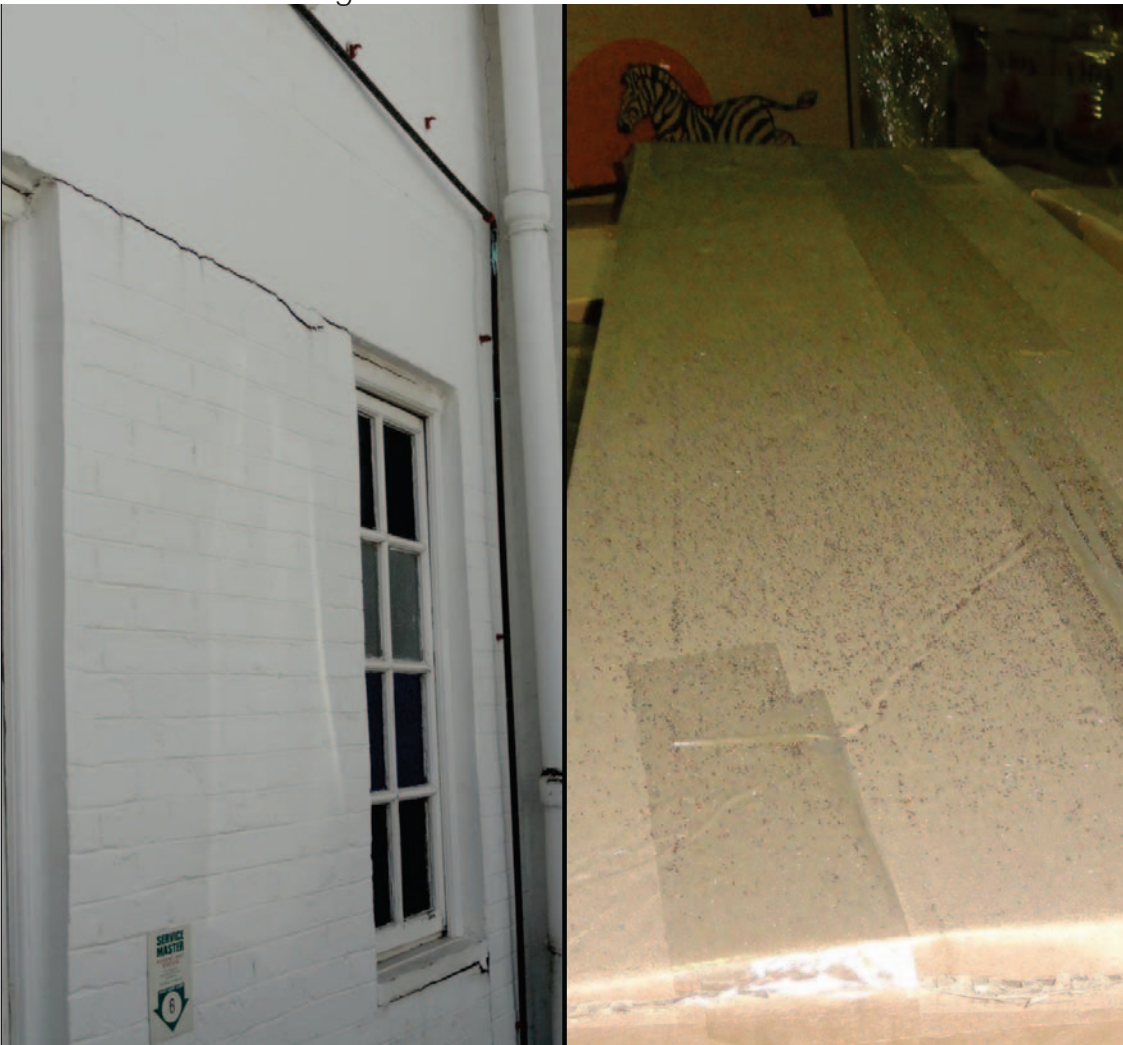
zone 03 | structural cracks and borer infestation
