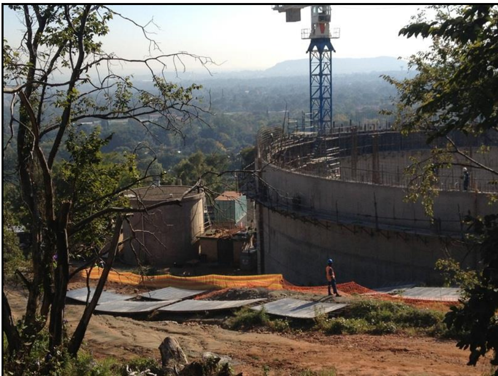
Figure 5: Infrastructure construction at the Annlin Reservoir site. The existing break pressure tank is visible to the right of the new reservoir structure.
