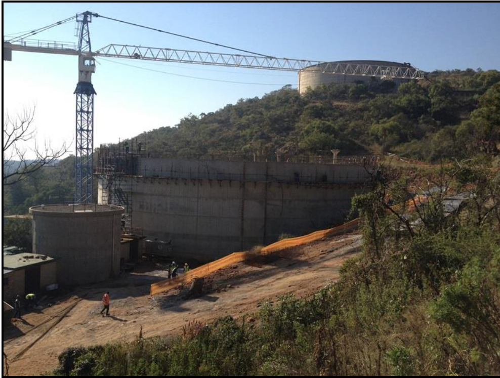
Figure 4: View of the Annlin Reservoir construction site along the western sector of the site. Note the existing Wonderboom Reservoir on the hill in the background.
