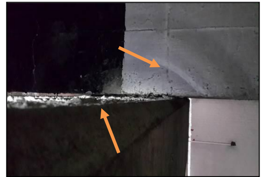
Photograph 3- Note gap between beams ~ 20 mm
