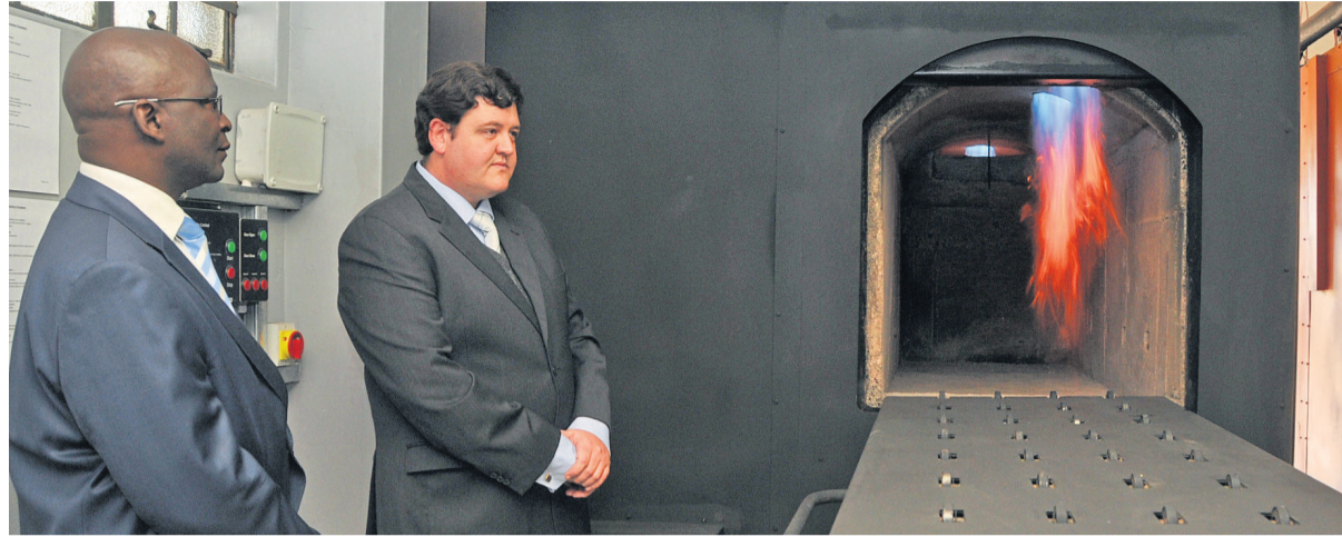
Msunduzi Mayor Chris Ndlela tests the new cremator at the Mountain Rise Cemetery at the handover by the contractors on August 16, 2013. With him is the contractor James Fairbrass, MD of SA Incinerator Company.
