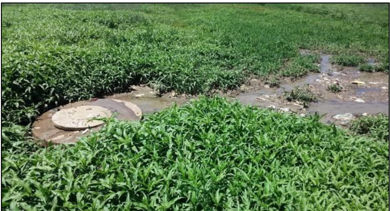
Figure 6: Sewage overflow from manhole on site creating a large wet area
