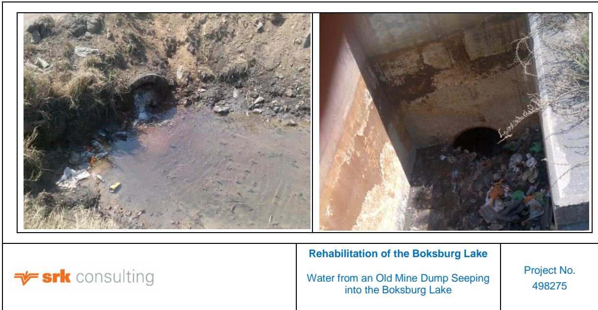
Figure 10: Water from Old Mine Dump seeping into the Boksburg Lake
