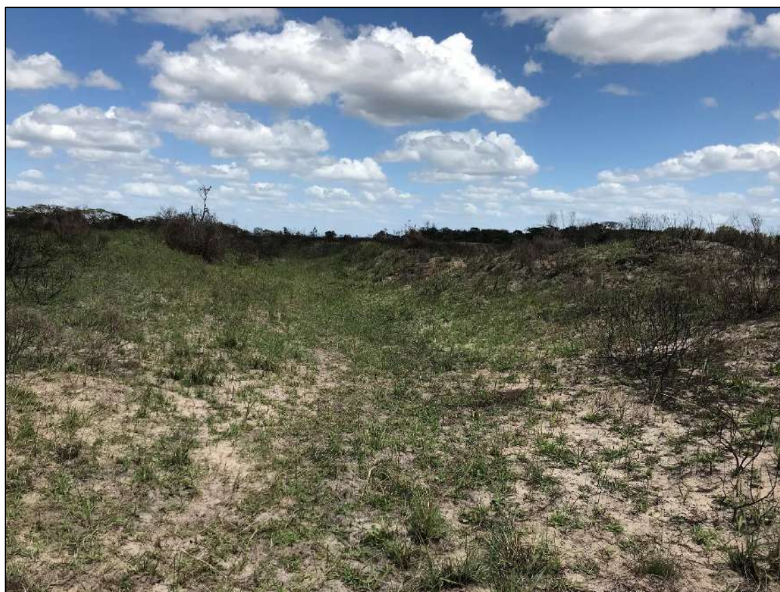
Figure 4.15 Photographic evidence of the excavated drain and the spoil deposits running along either side of the drain.
