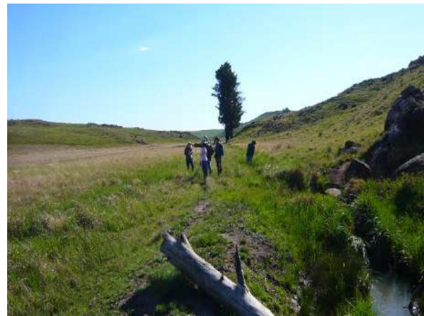
The main drain in the system that will be deactivated. The berm adjacent to the channel will be removed where necessary
