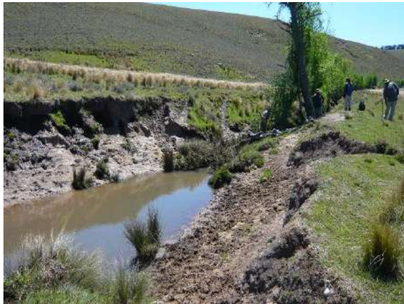
Damage to the banks of the main channel caused by livestock crossing.
