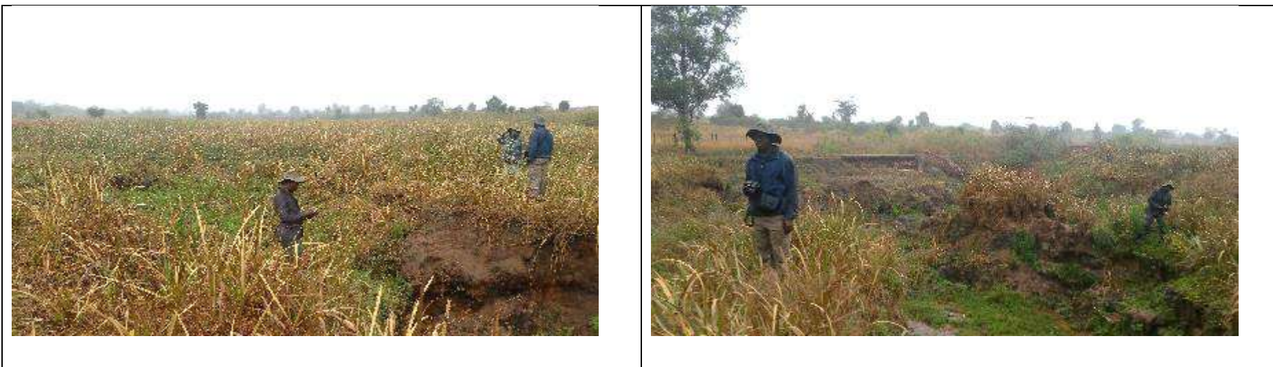
Figure 9: Photos of the site depicting the extent of the erosion
