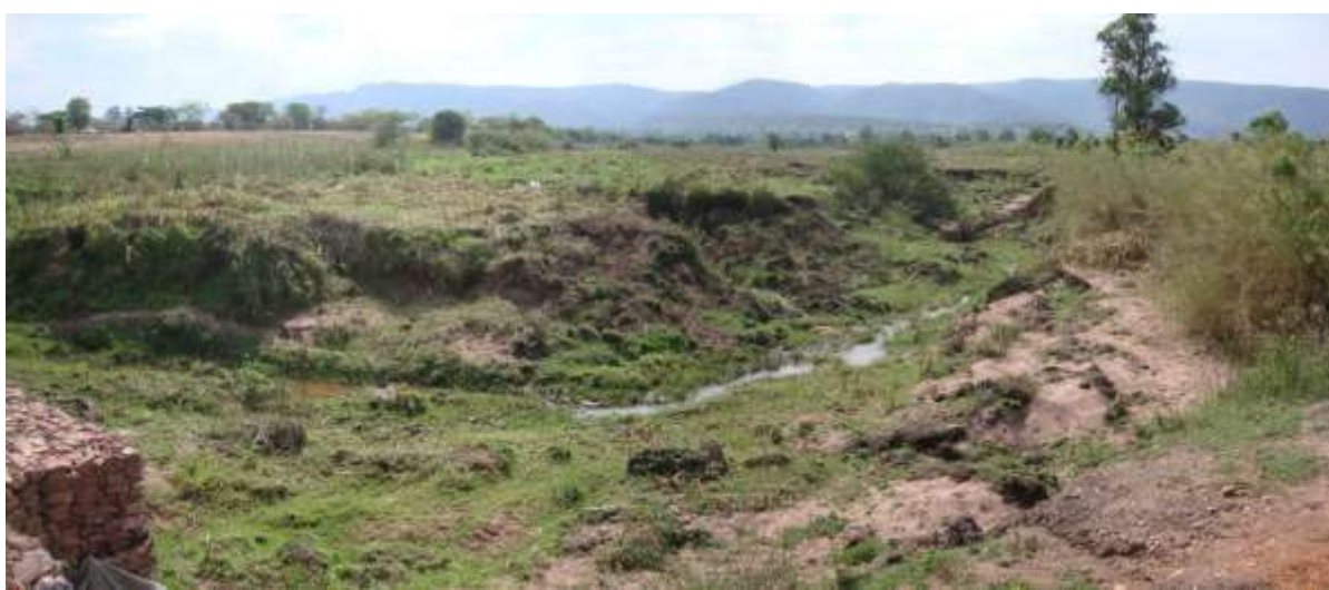
View downstream of an existing rehabilitation weir that is currently threatened by active erosion.
