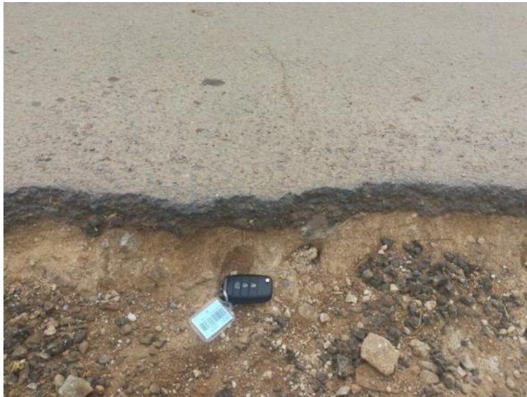
Photo 15: Edge drops between Maple Street - EP Malan Street
