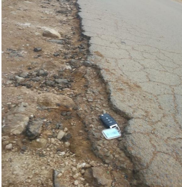
Photo 16: Edge drop resulting from scouring of the gravel shoulder
