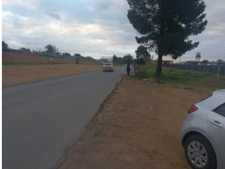
Photo 14: Edge breaks between Maple Street - EP Malan Street
