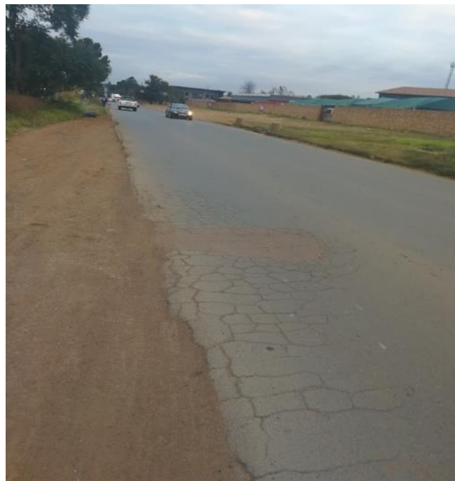
Photo 6: Pumping on the wheel path between Maple Street - EP Malan Street
