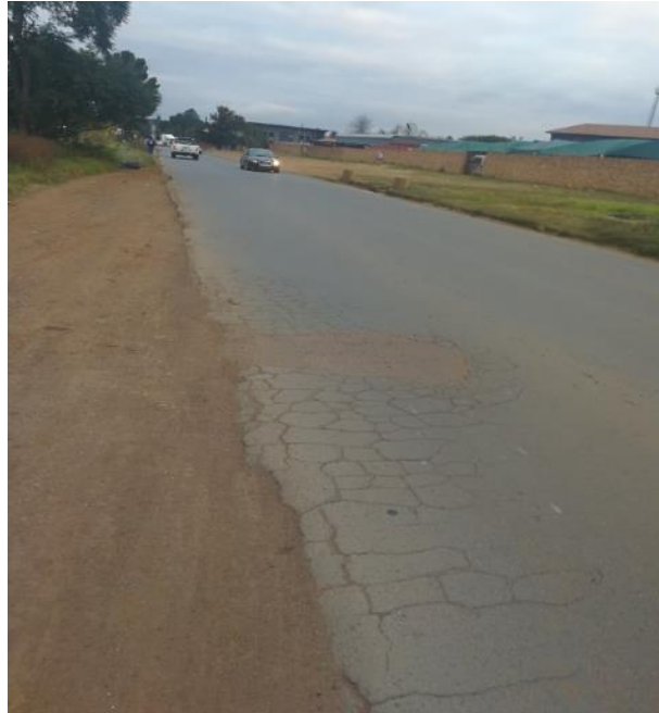
Photo 13: Patchwork on the wheel path where rutting and crocodile cracking have advanced between Maple Street - EP Malan Street
