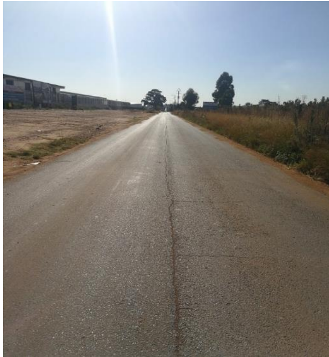
Photo 5: Longitudinal cracks between Deodar Street and West Street
