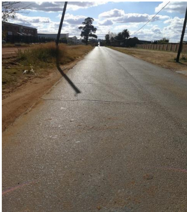
Photo 2: Block cracks between Deodar Street and West Street
