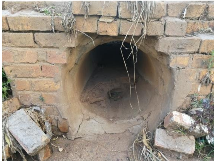
Photo 19: blocked culvert pipes at the small stream
