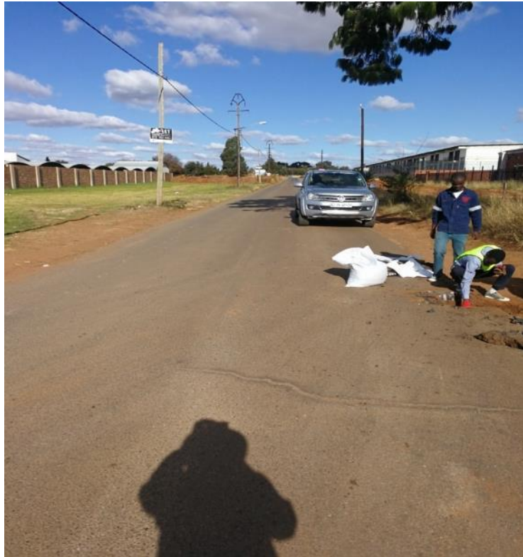
Photo 1: Transverse crack between Deodar Street and West Street
