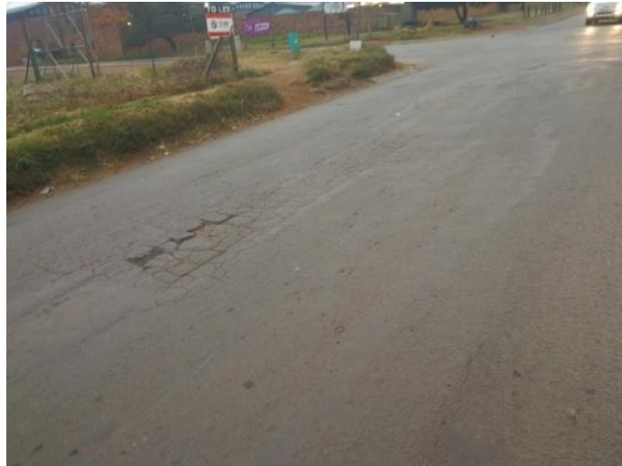
Photo 7: Surface failure between EP Malan Street and Elgin Street
