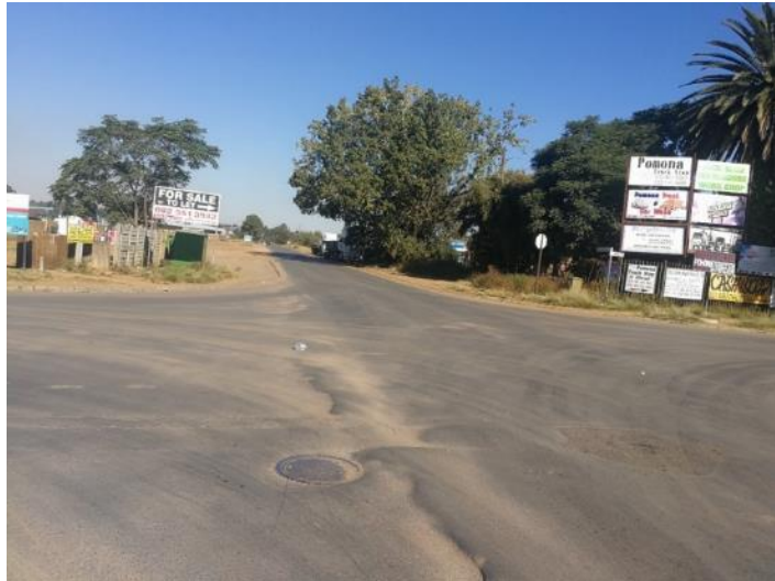
Photo 9: Shoving of surfacing at Maple Street
