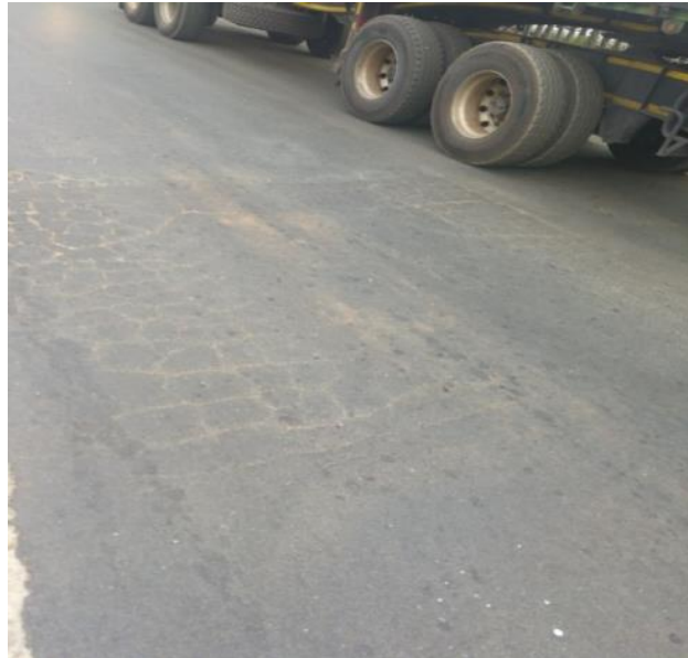
Photo 3: Crocodile cracking between Pomona Road - Maple Street
