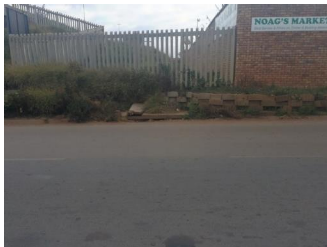
Photo 18: Blocked kerb inlet between Pomona Road - Maple Street
