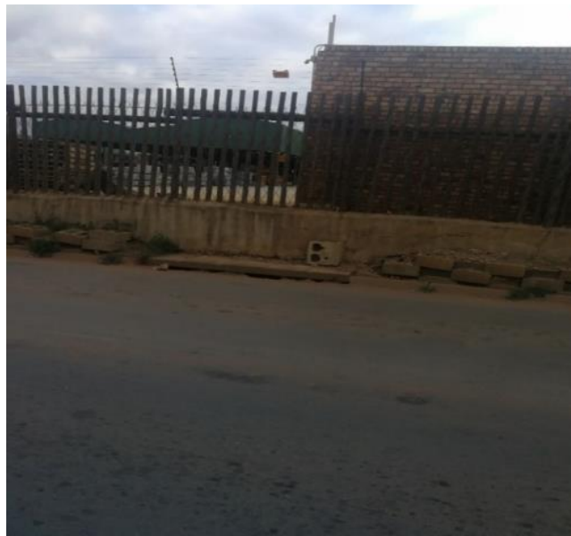
Photo 12: Slight bleeding on the wheel path
