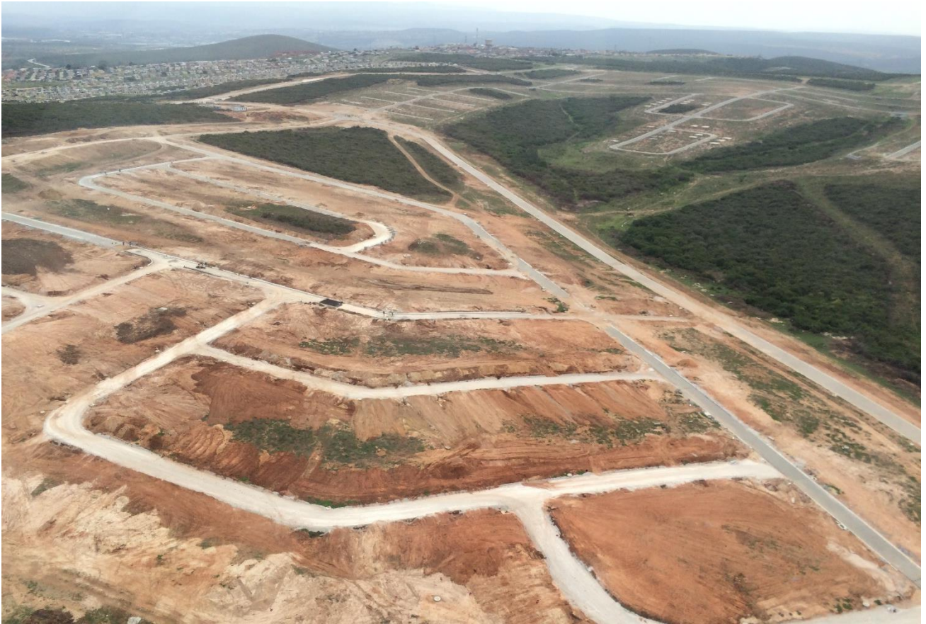
Figure 54: Aerial image of land cleared for the construction of housing developments next to Kwanobuhle (source: Palmer, 2017)
