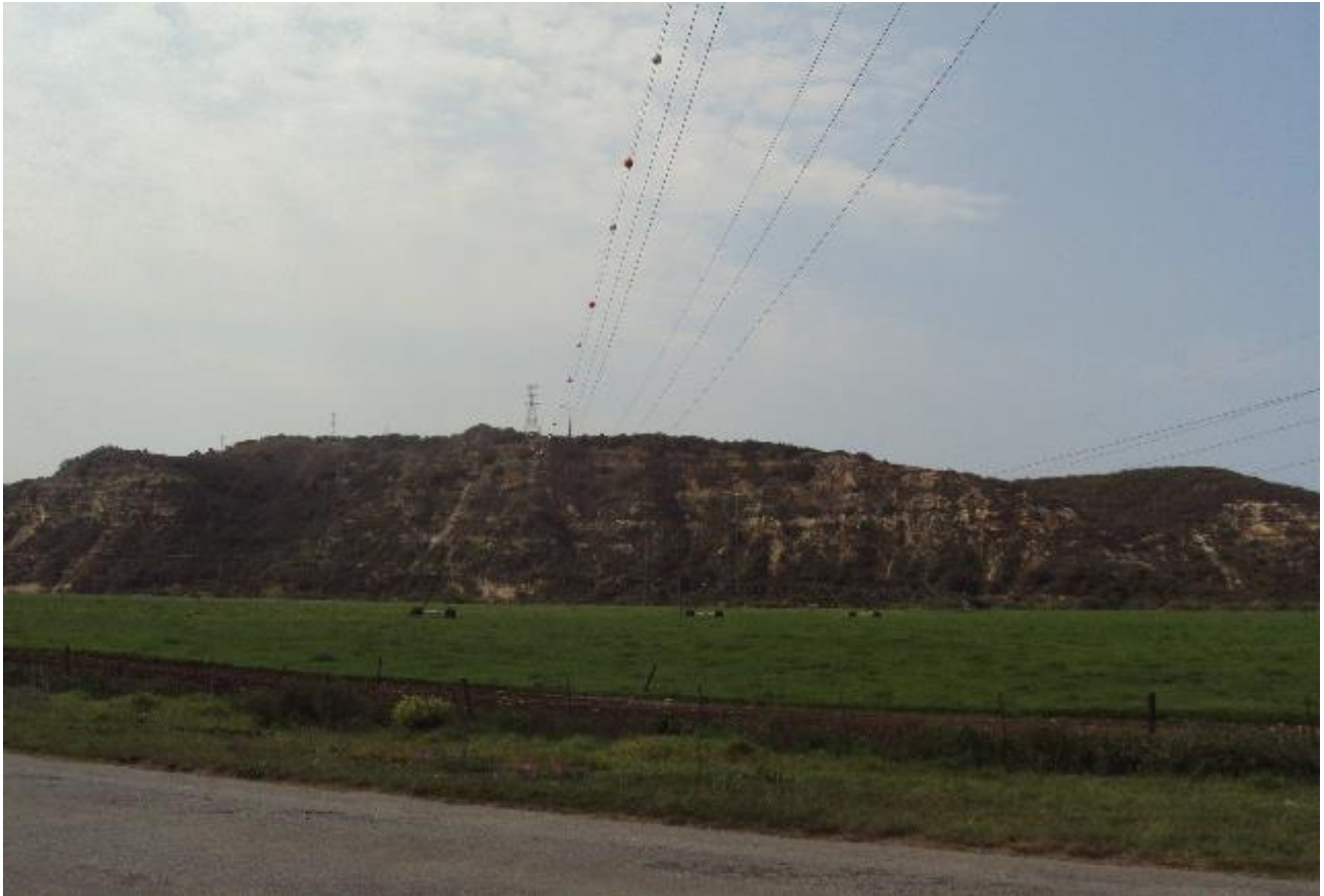
Figure 51: Existing Eskom 132kV overhead powerline running up the steep climb across the Gamtoos River visible from R102
