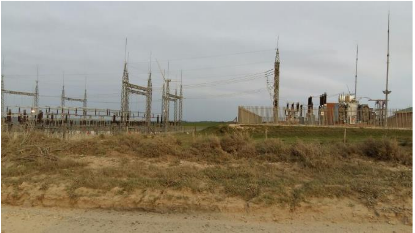
Figure 20: Example of a substation and switching station on the Kouga Wind Farm
