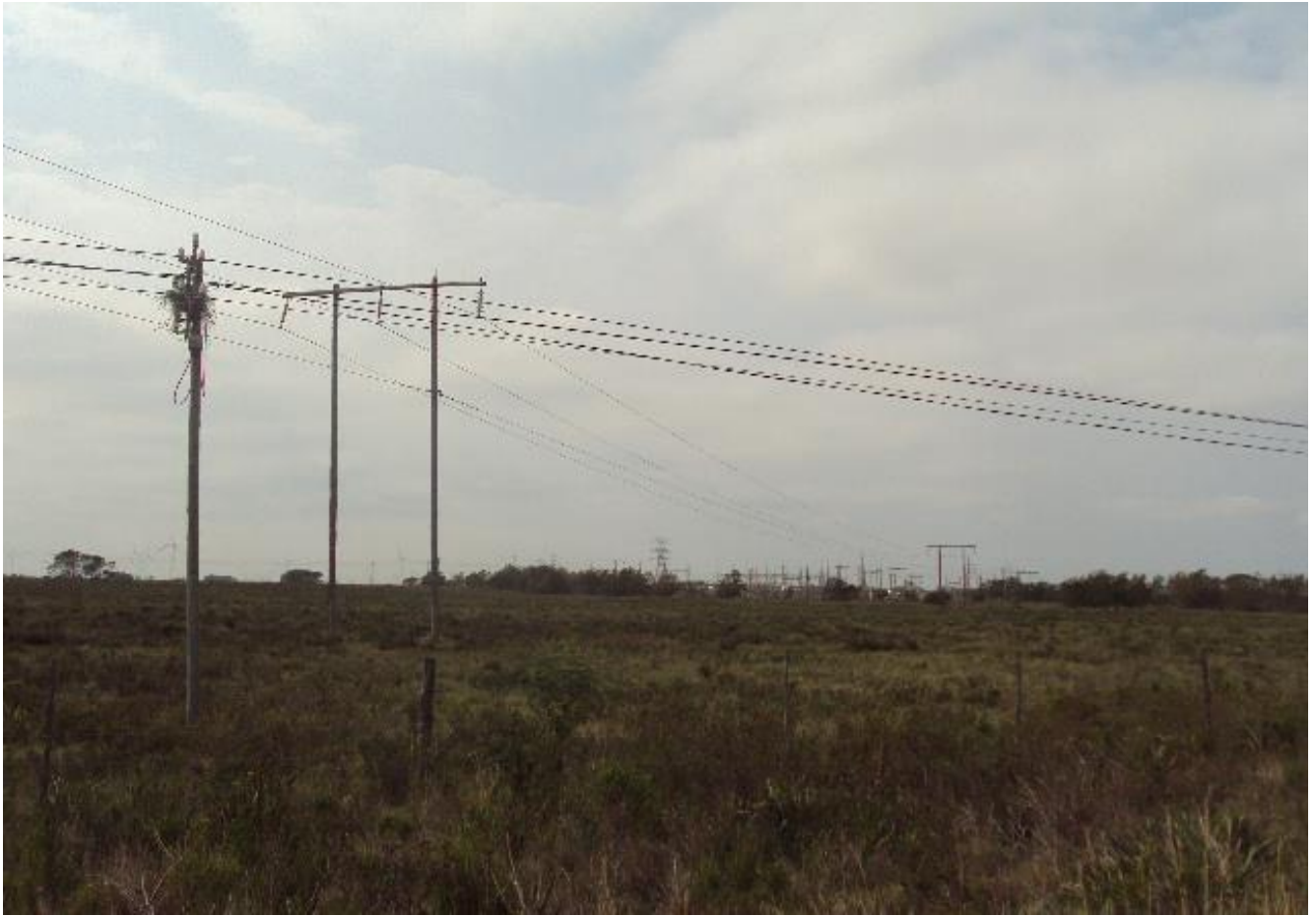
Figure 49: Photograph of existing 66kV overhead powerline and telephone line, with Melkhout substation in the background approximately 500 m away (source: Jones, 2017)
