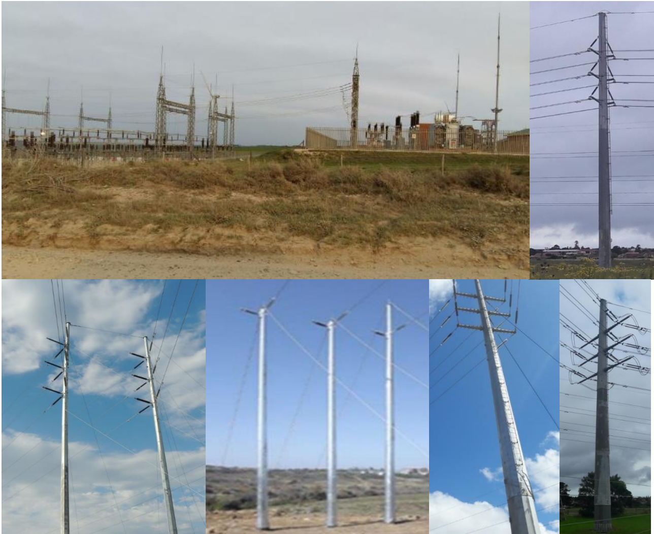
Figure 2: Examples of the main types of pylons to be used and of a switching station (see BAR for detail)
