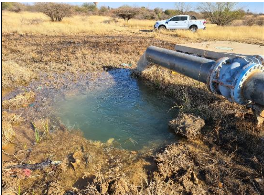
Photograph 8. Leaking pipeline in the north-eastern section of the Roodepan site
