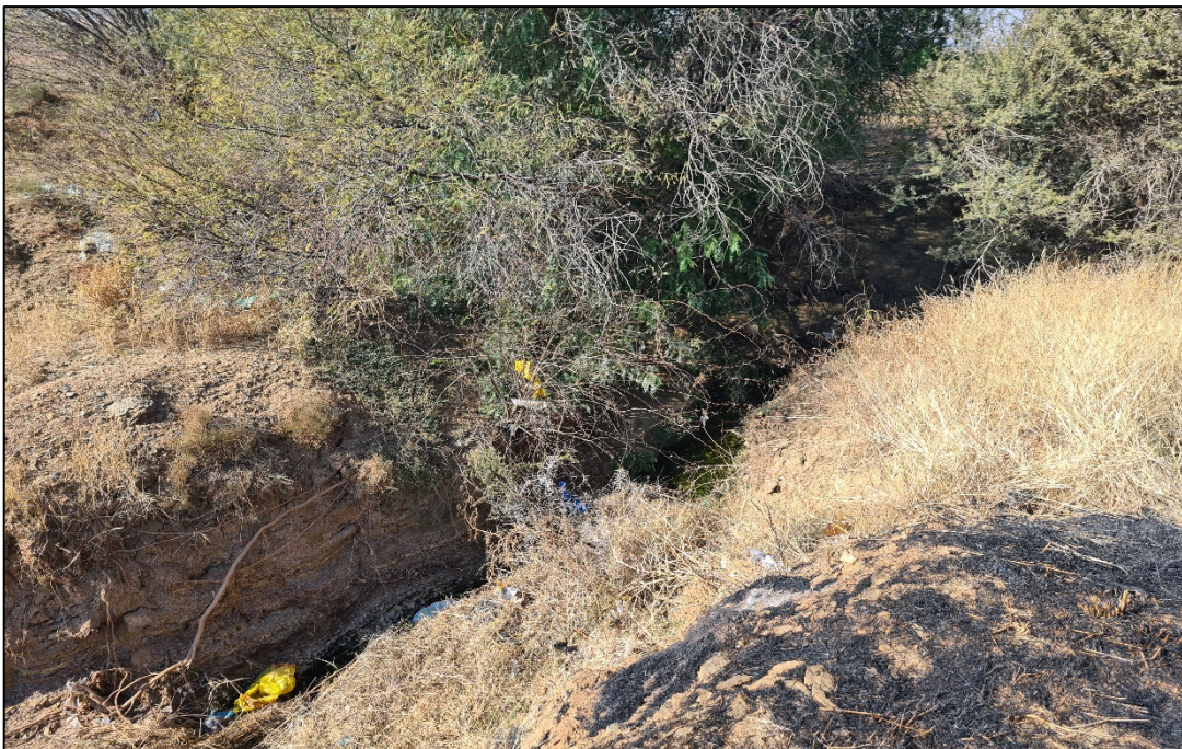
Photograph 9. Highly eroded stormwater canal that feeds the quarries in the project area
