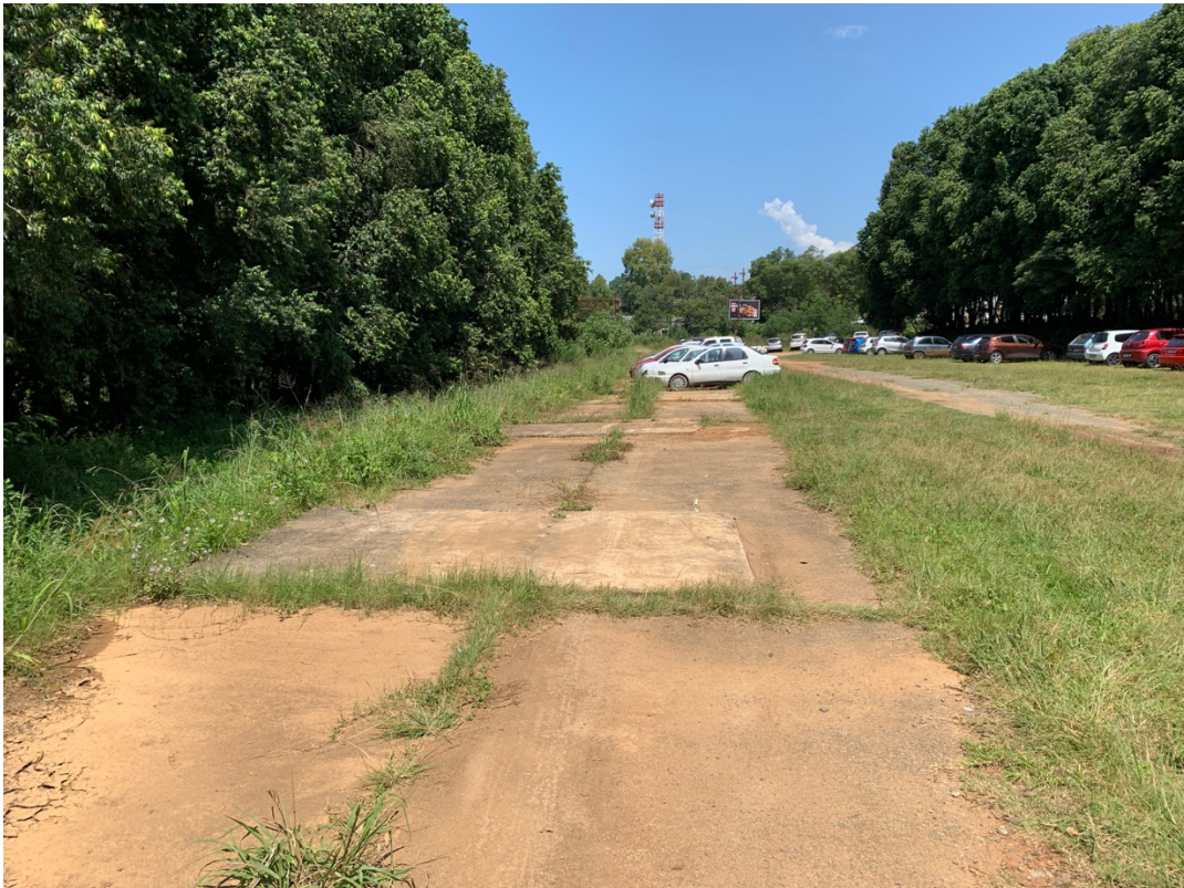
6- The concrete hard stand: view towards the south from the northern end of the siding
