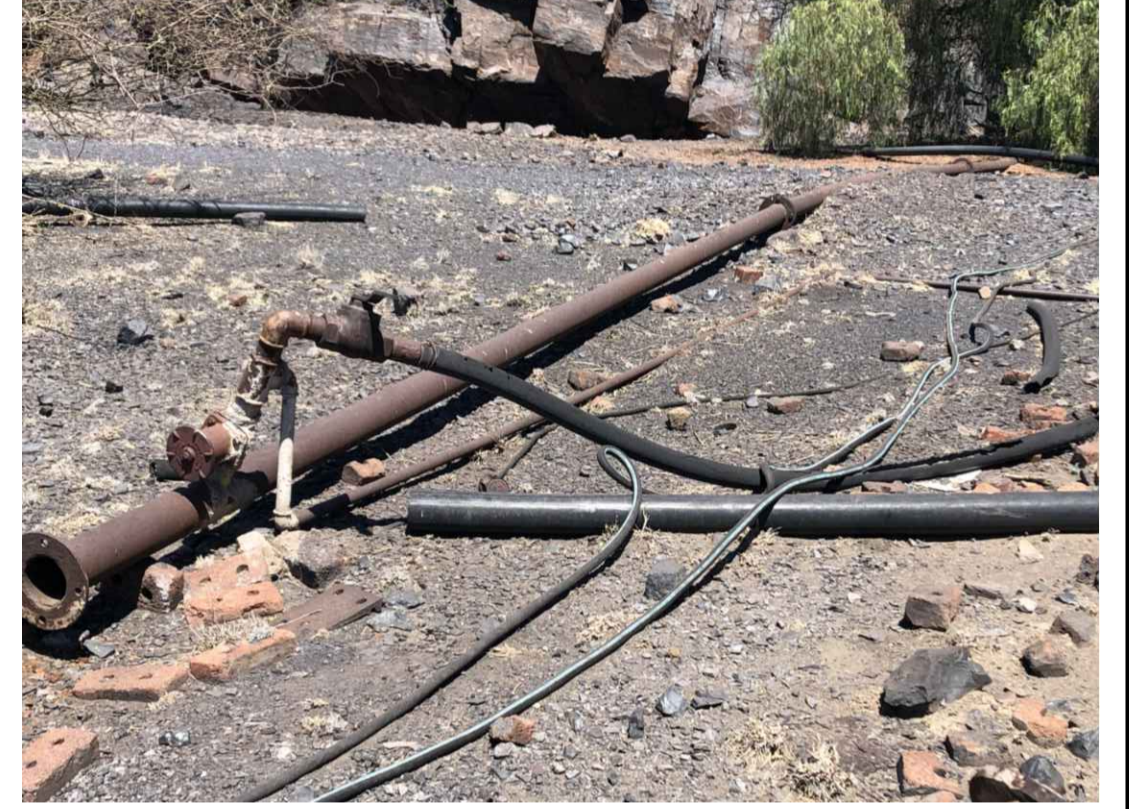
OLD DISUSED PIPES
