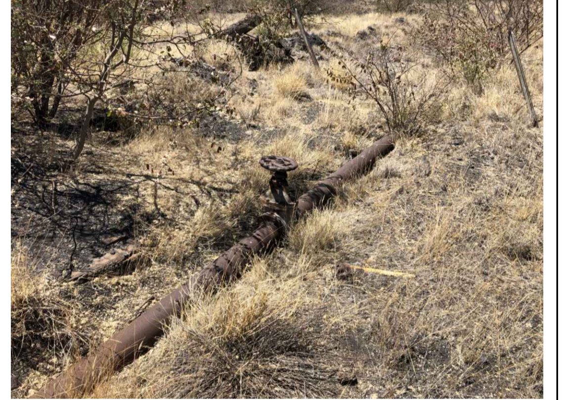
OLD DISUSED PIPES
