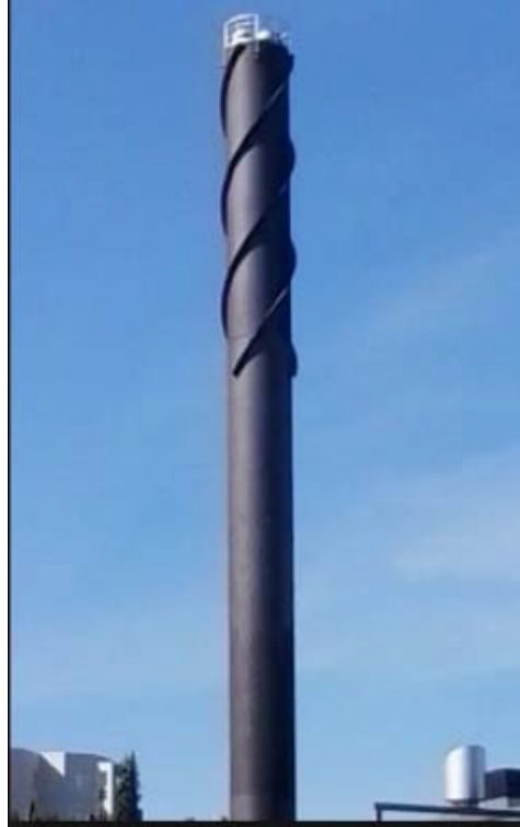
Boiler stack with helical strakes to limit vibration associated with wind induced periodic vortex shedding
