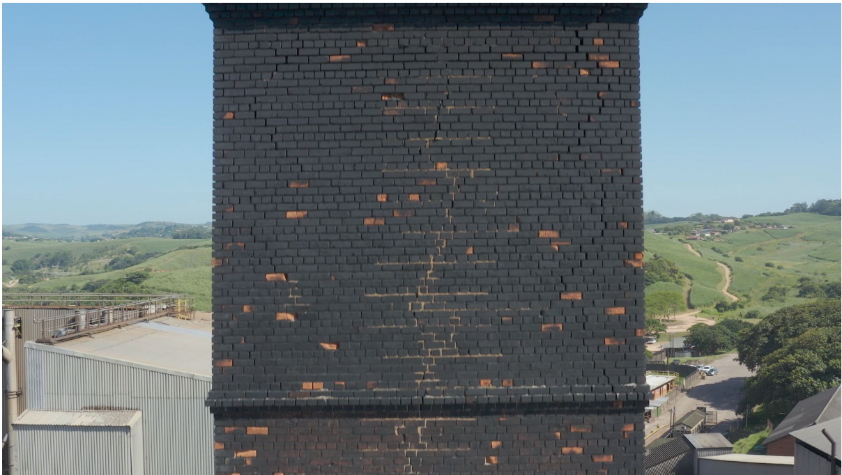
Eastern Facing Cracking
