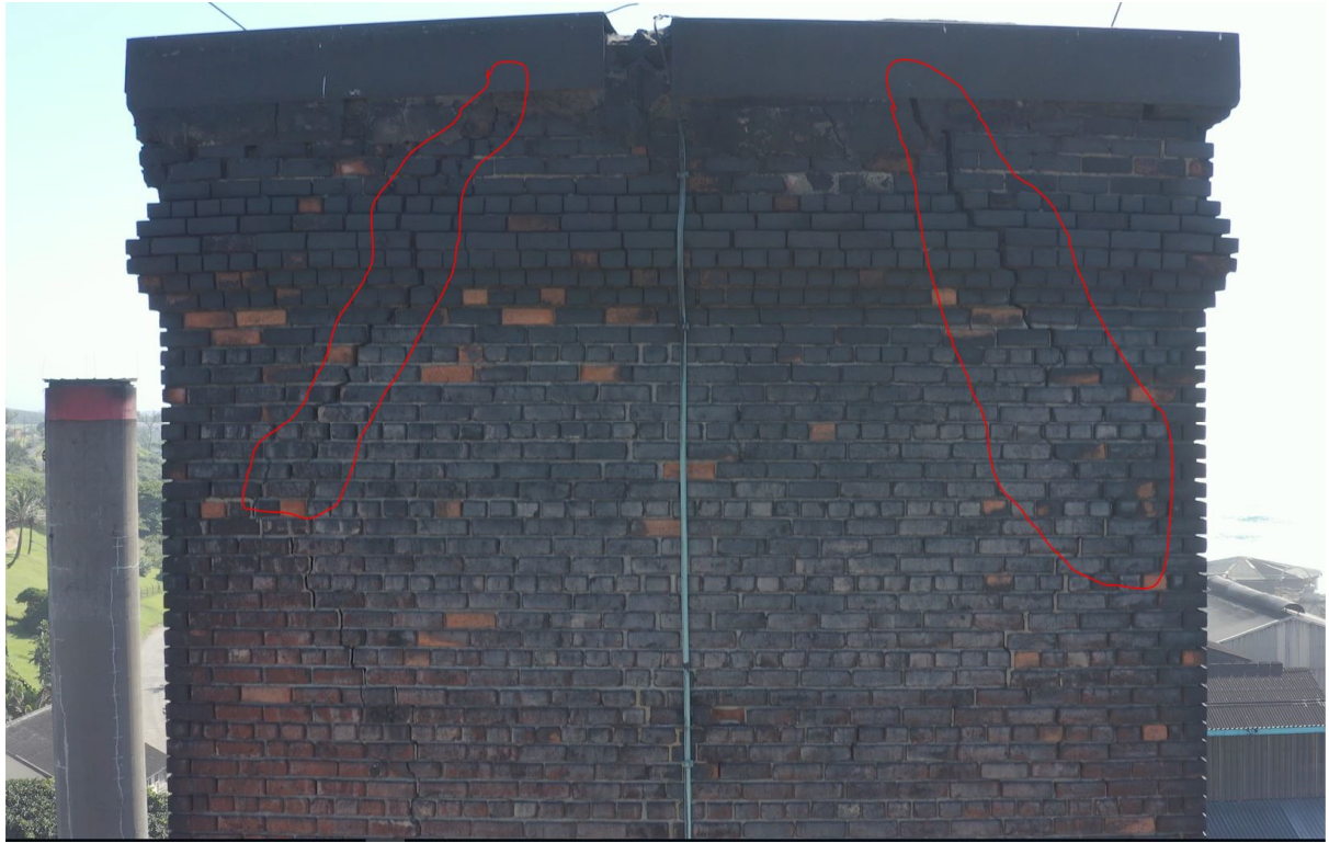
Southern Facing Cracking
