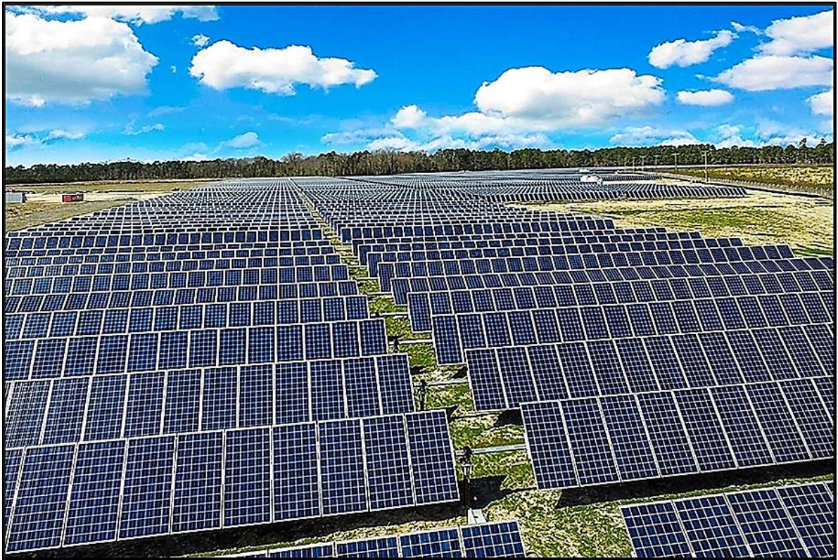
Figure 2.1: Typical example of solar PV array
