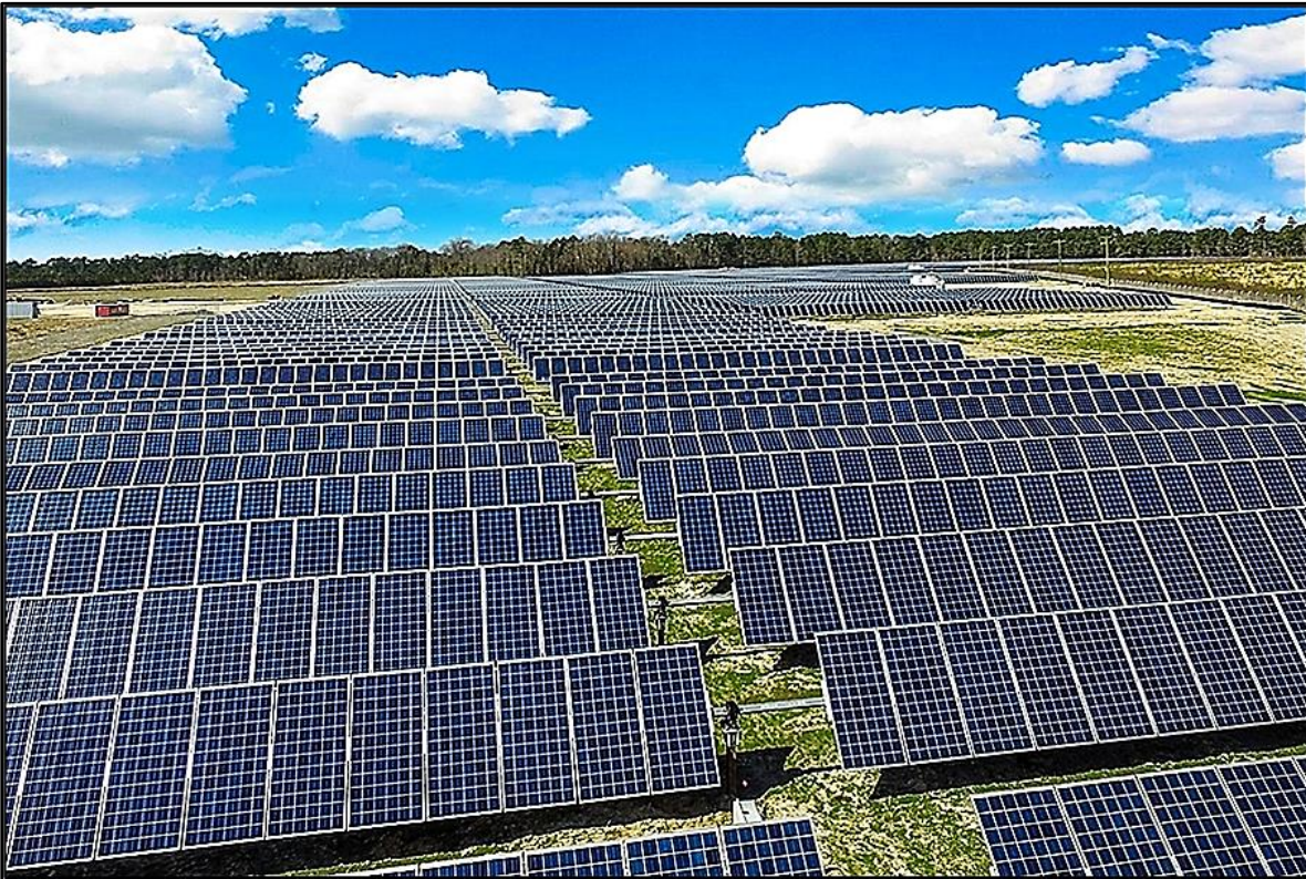
Figure 2.1: Typical example of solar PV array
