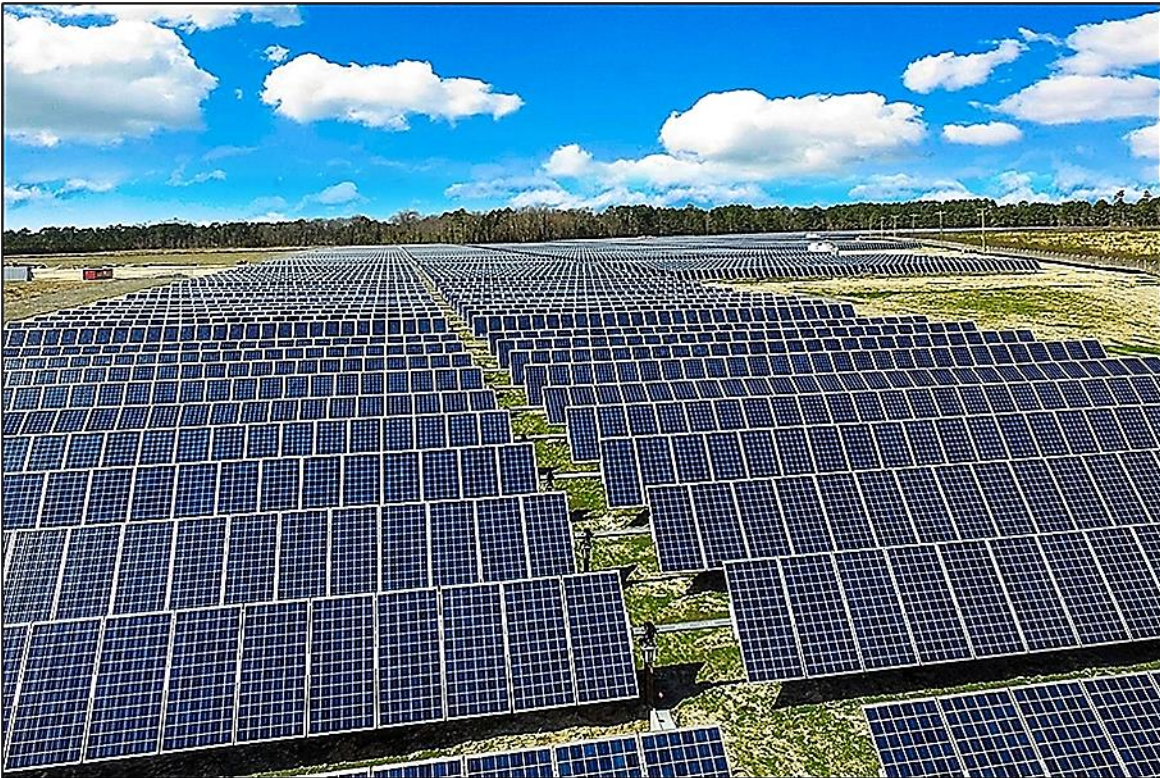
Figure 2.1: Typical example of solar PV array
