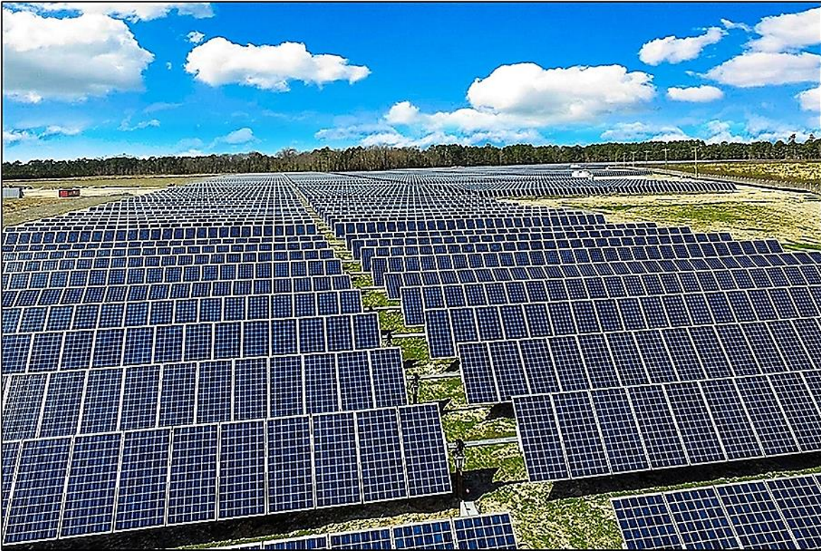
Figure 2.1: Typical example of solar PV array
