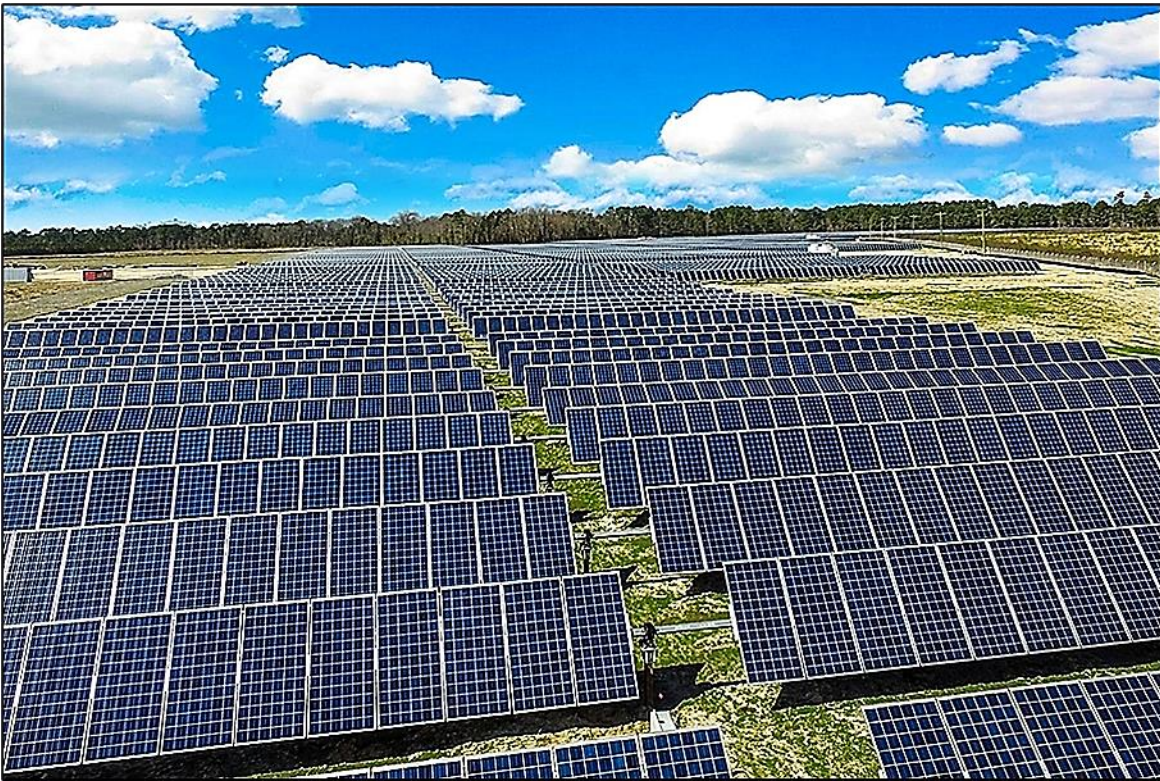
Figure 2.1: Typical example of solar PV array
