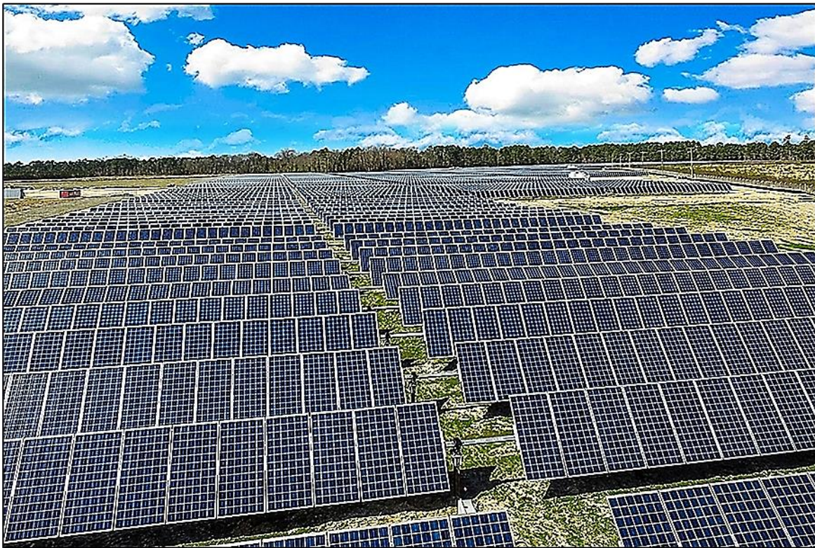
Figure 2.1: Typical example of solar PV array
