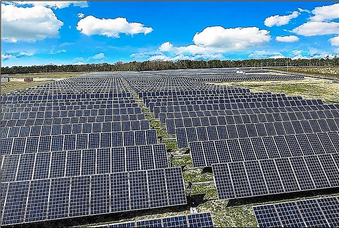
Figure 2.1: Typical example of solar PV array
