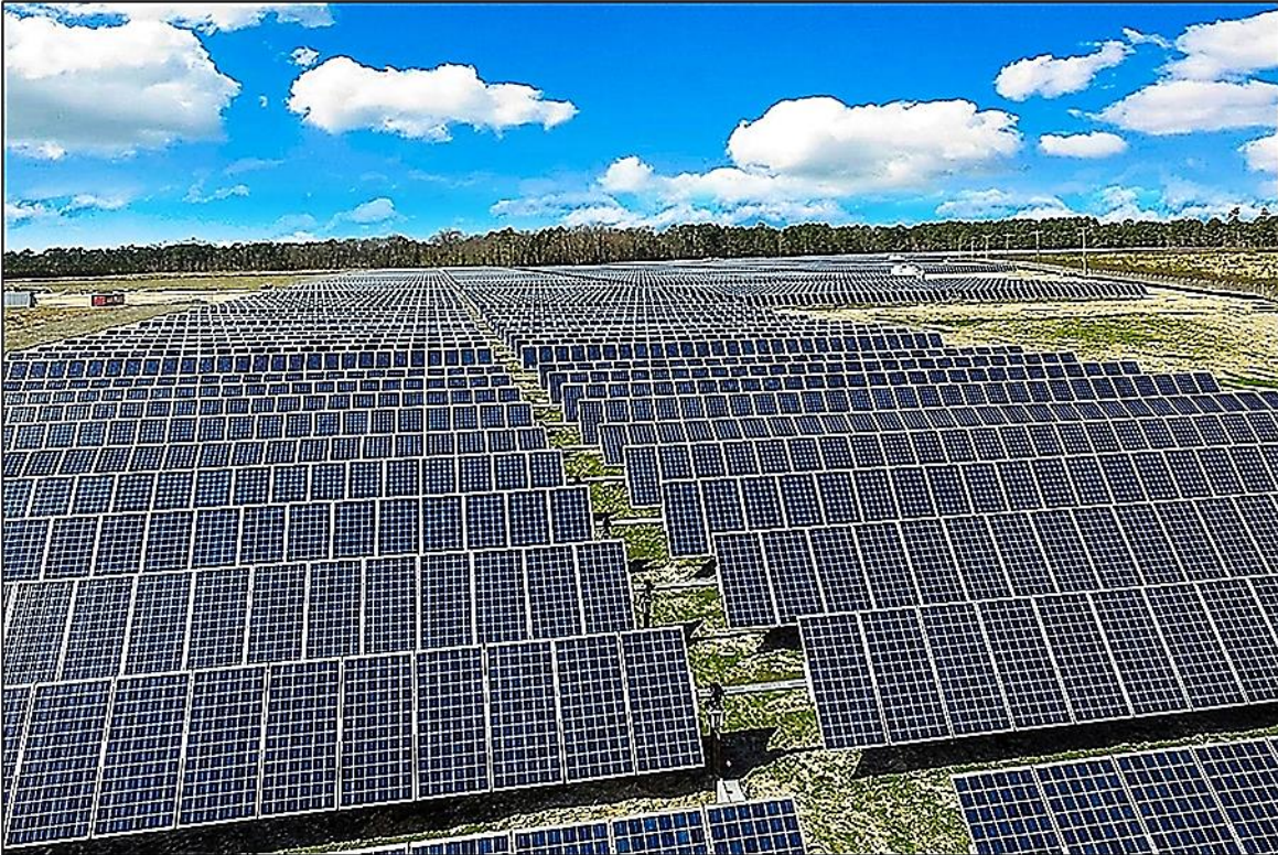
Figure 2.1: Typical example of solar PV array
