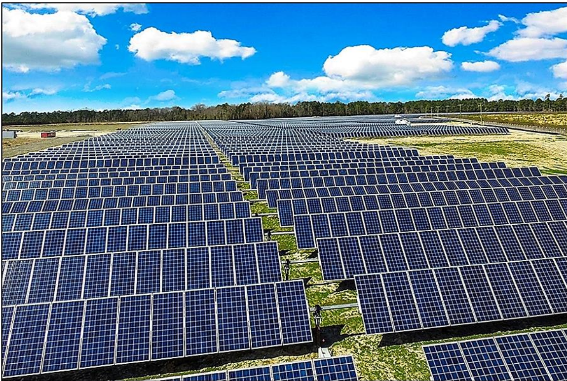
Figure 2.1: Typical example of solar PV arrays
