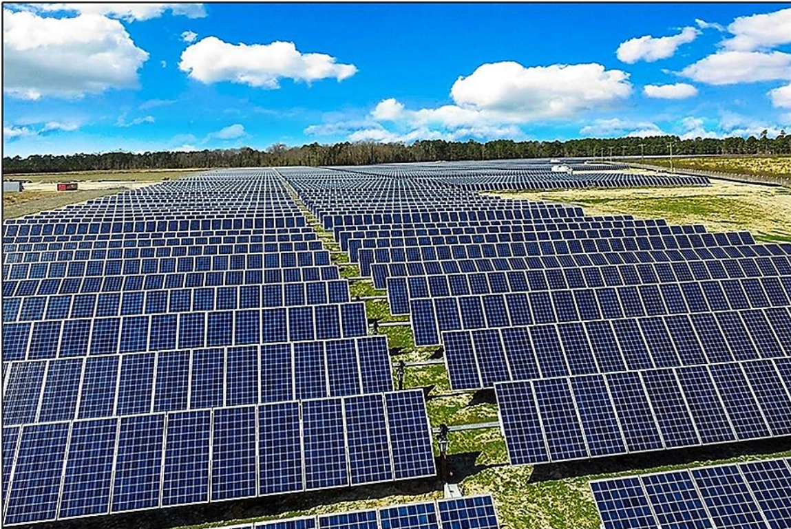
Figure 2.1: Typical example of solar PV arrays
