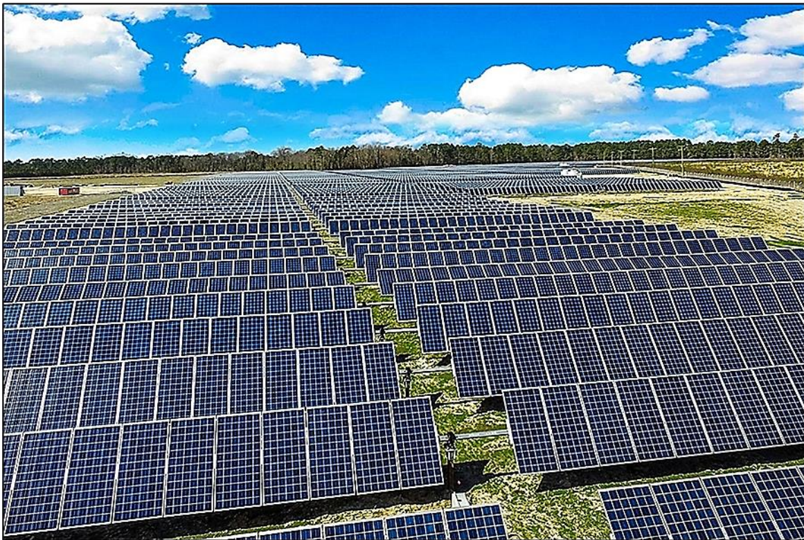
Figure 2.1: Typical example of solar PV array
