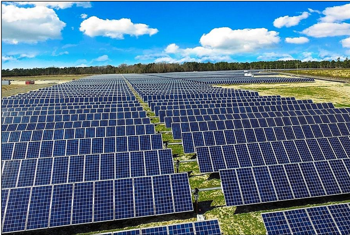
Figure 2.1: Typical example of solar PV array
