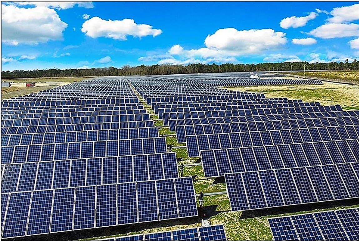
Figure 2.1: Typical example of solar PV arrays
