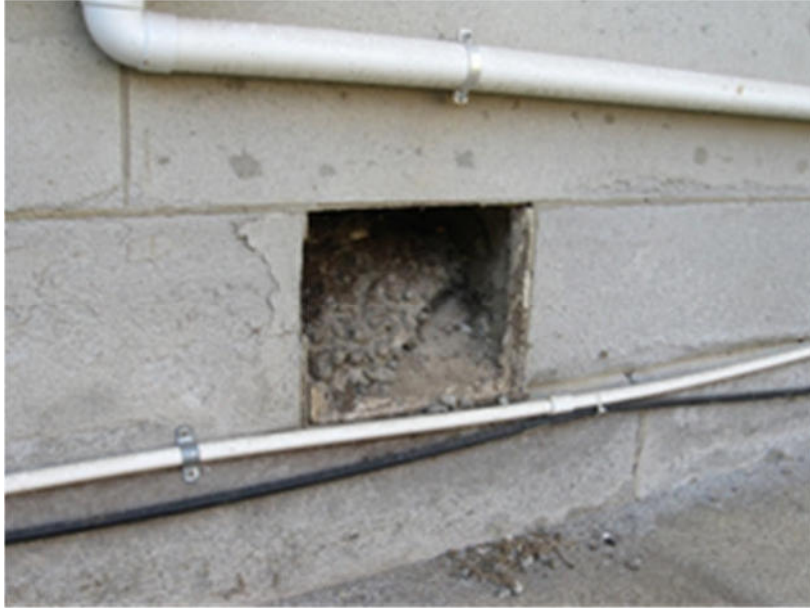
Damaged floor vent
