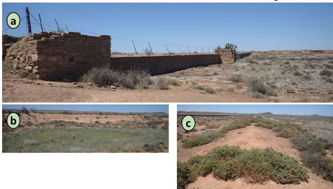
Figure 43: A visual compilation of the Brak River crossing and upstream dam. a) Rock wall dam b and c) earth fill dam wall and berm.
