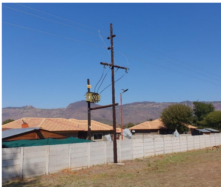
Figure 6 Typical Pole Mounted Transformer
