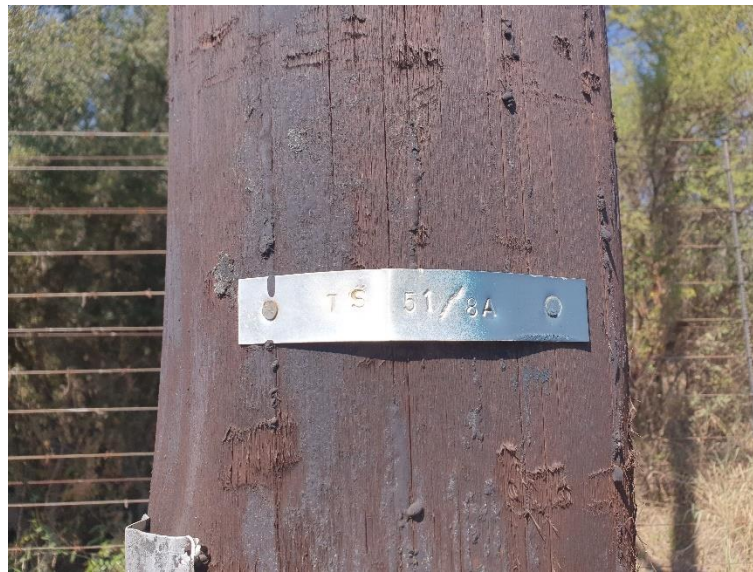
Figure 4 Pole TS 51/8A
