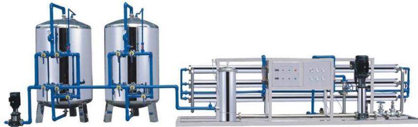
Figure 3 Example of a water treatment plant (EcoPura RO Plant)
