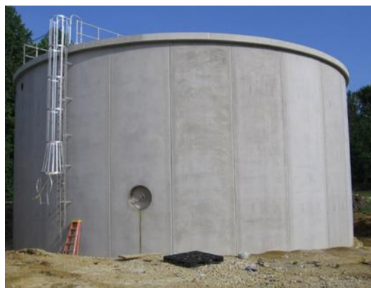
Figure 2 Typical water reservoir
