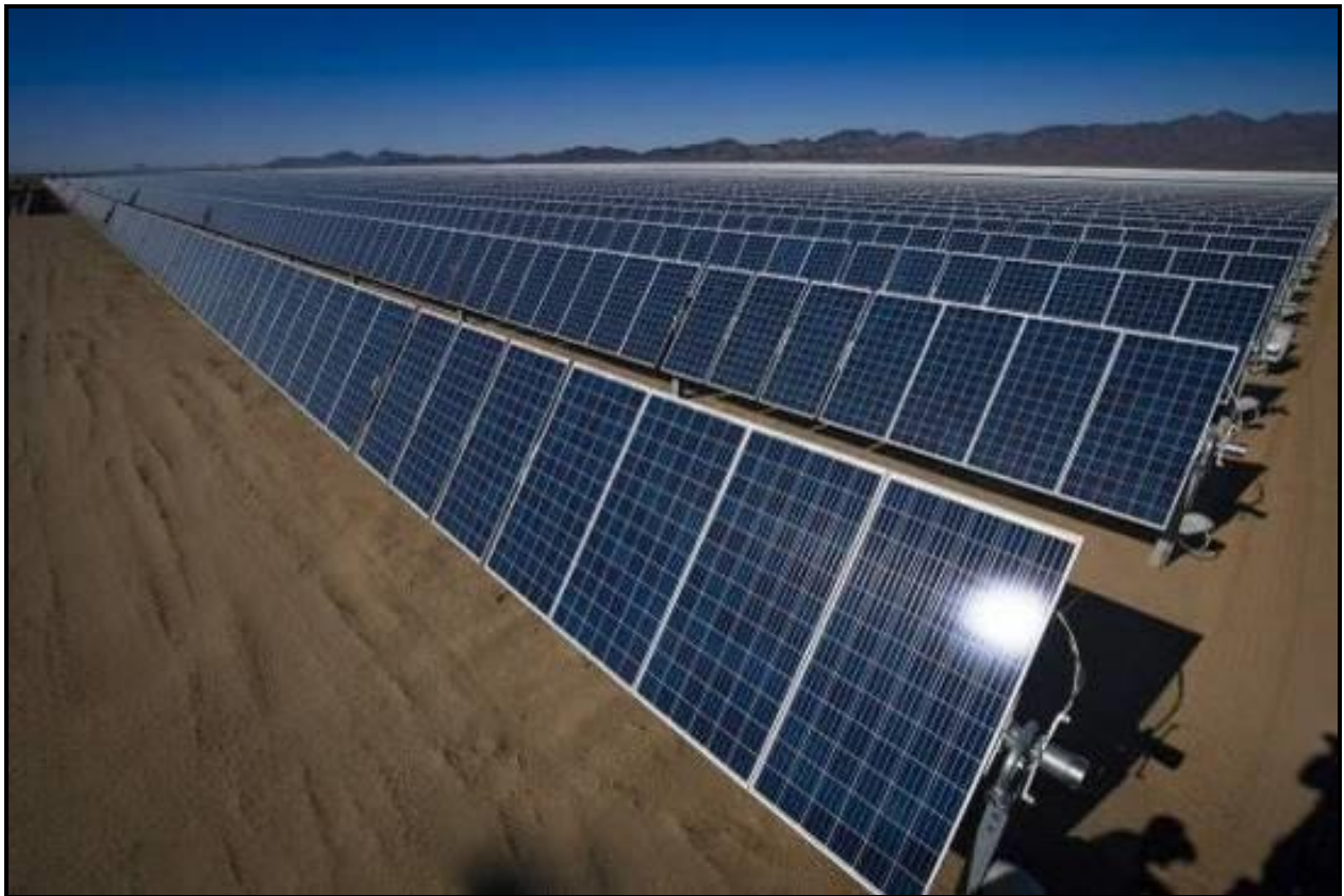
Photograph 1.1: Typical PV SEF facility
