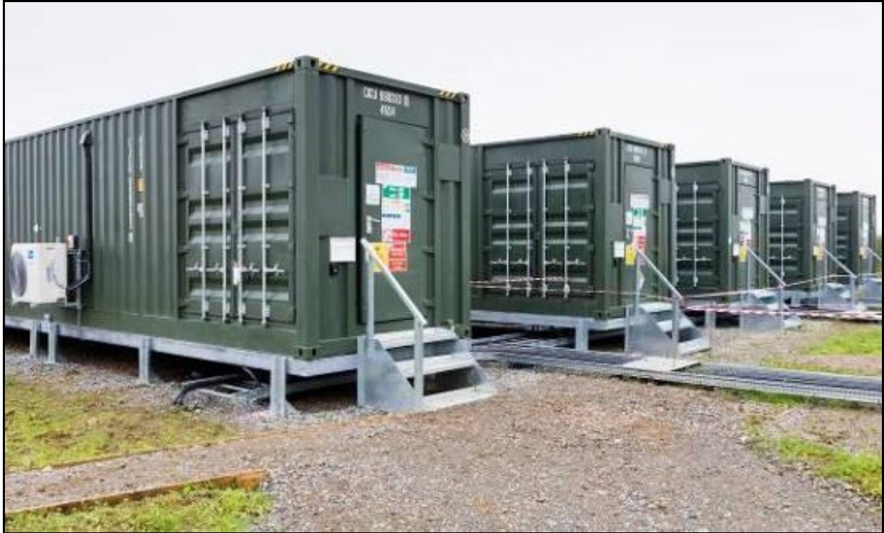
Photograph 1.2: Example of BESS located in storage containers
