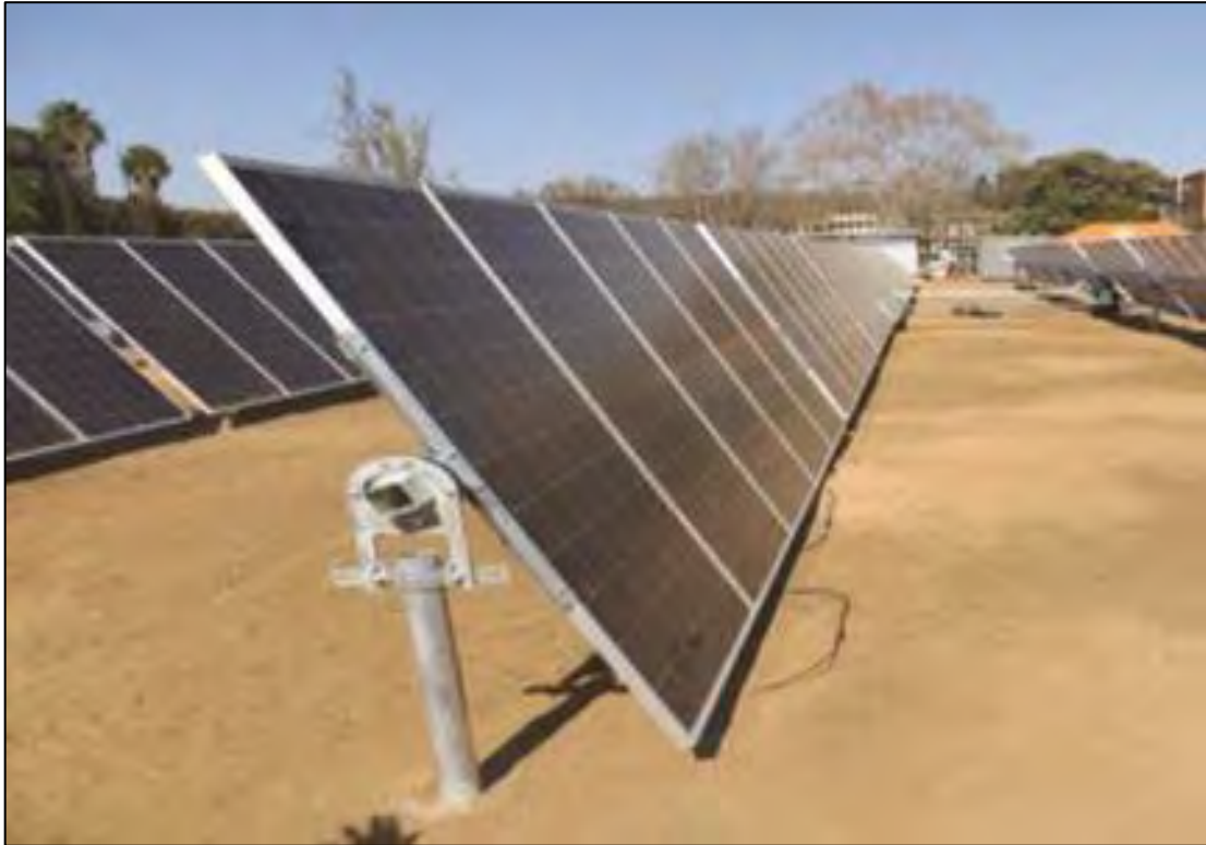
Plate 1-2: Single axis solar PV module tables raised 1.5m above ground level (to a maximum tilt height of 3m).
