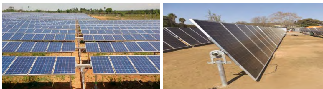
Figure 4-1: Single axis solar PV module tables raised 1.5m above ground level (to a maximum tilt height of 3m)
