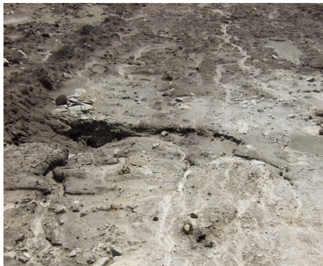
Figure 4: Slight collection of water which will result in soil material being washed into the void
