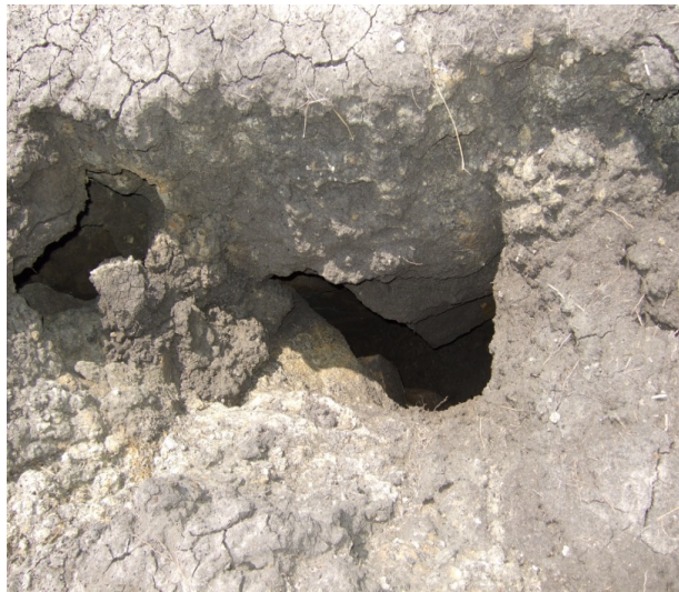
Figure 3: Crack where fill material was washed into the void
