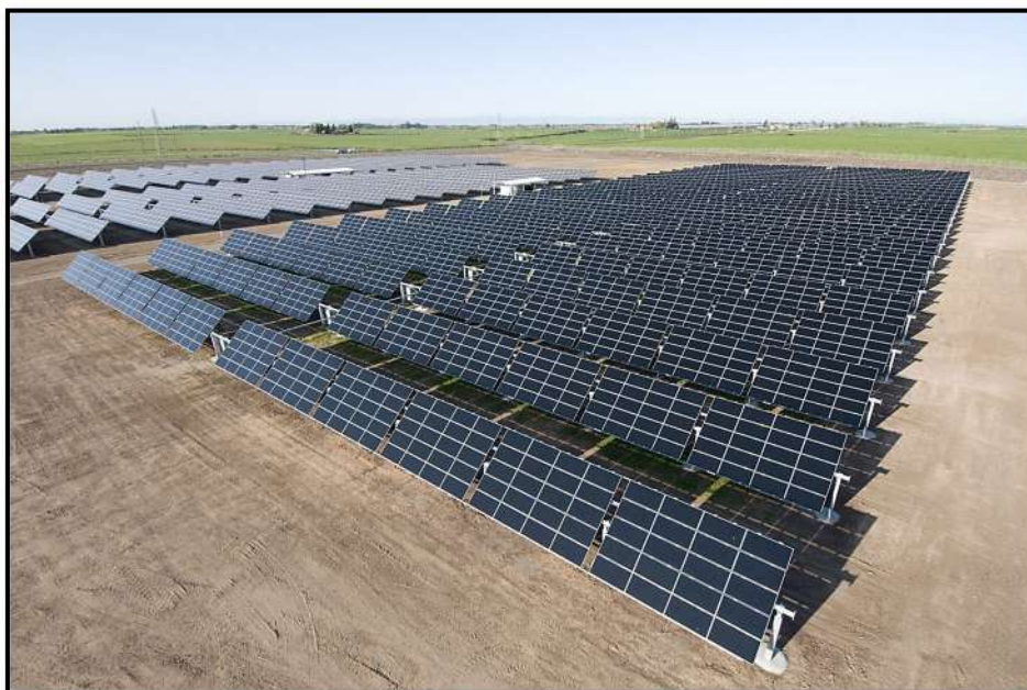
Photographs 5.2.2 and 5.2.3: The photos above and to the right show a typical example of the mounting structure for a tracking PVSEF and an array of photovoltaic panels once mounted
