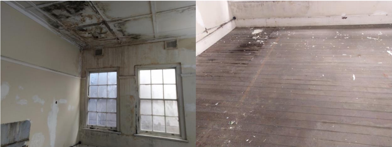
Figure 7: Ceiling water damage and floor fire damage on first floor
