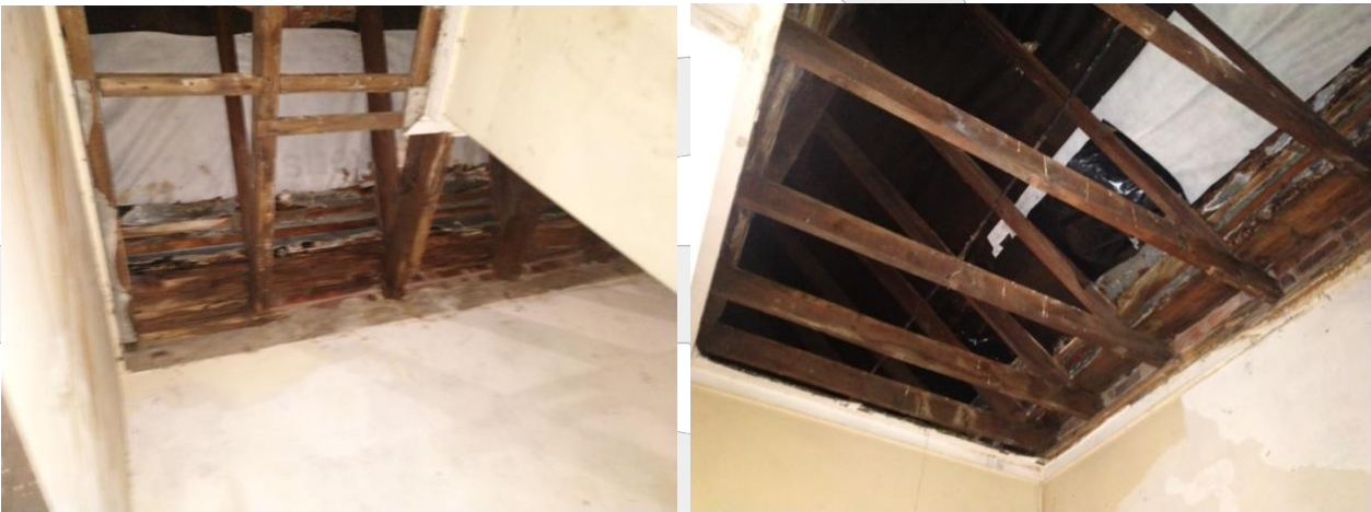
Figure 10: General condition of roof trusses and damage noted
