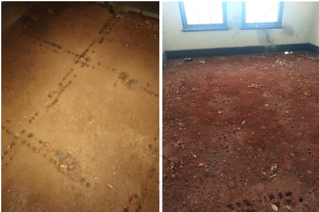
Figure 5: Traces of water ingress on ground floor
