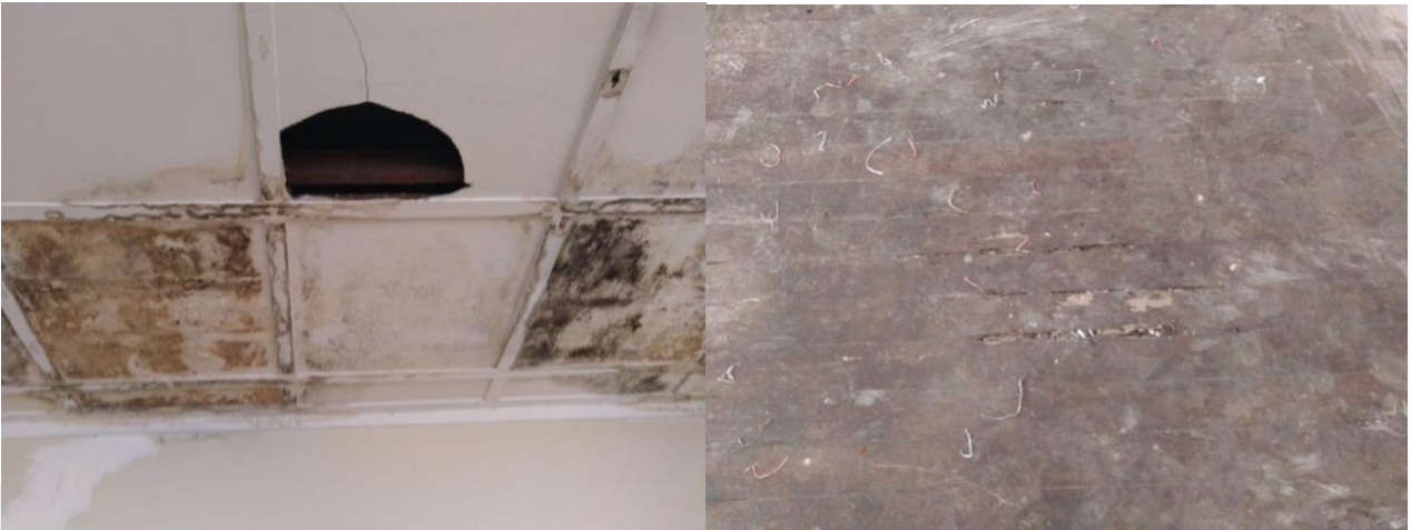
Figure 9: Ceiling damage and floor damage on the first floor
