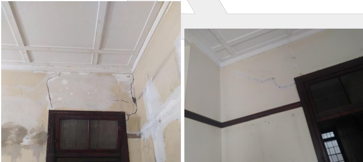
Figure 4: Cracks over the ground floor doorways
