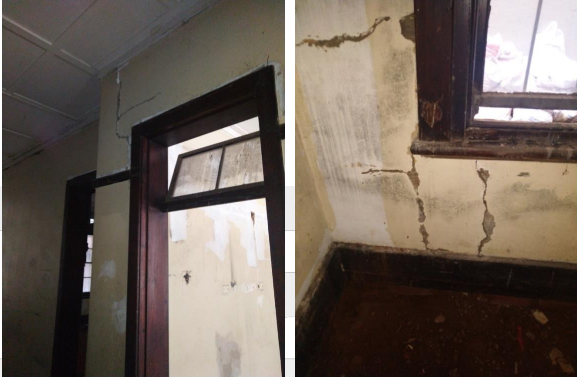
Figure 3: Cracks on ground floor doorways and windows
