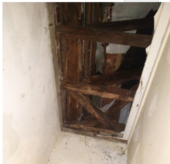
Figure 11: Water damage and wood rot observed in certain areas of trusses
