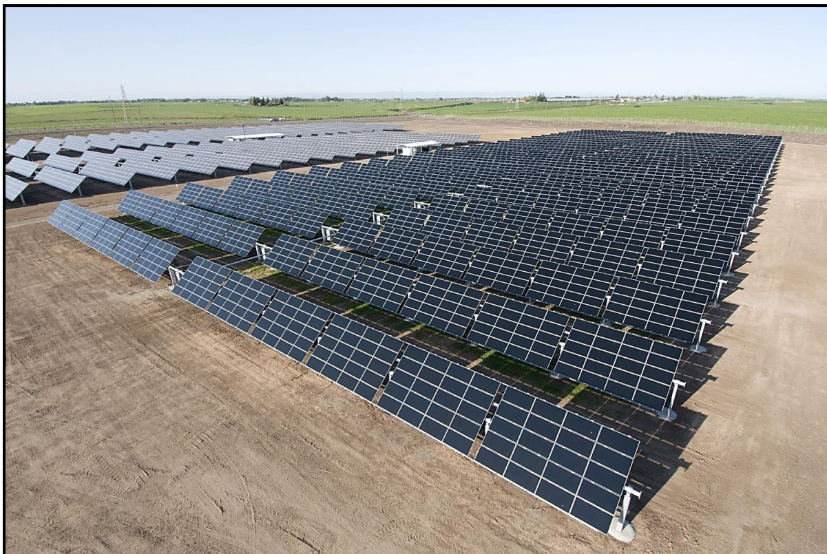
Figure 19: An array of mounted PV Panels
