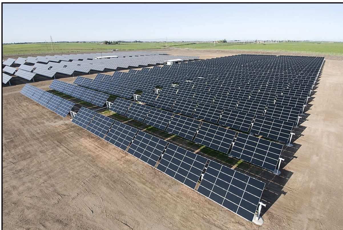
Figure 19: An array of mounted PV Panels
