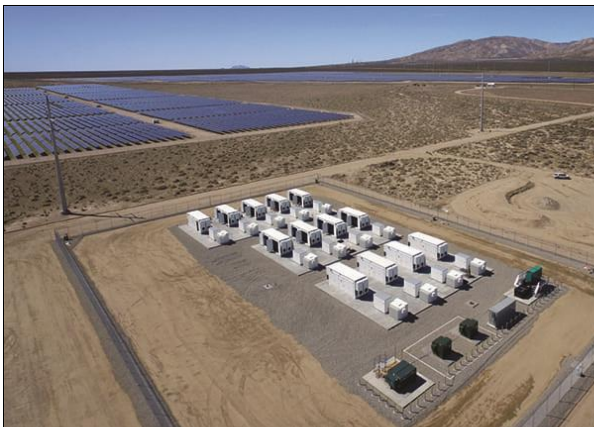
Figure 22: Example of a BESS (Beacon Solar Plant Site, LADWP)
