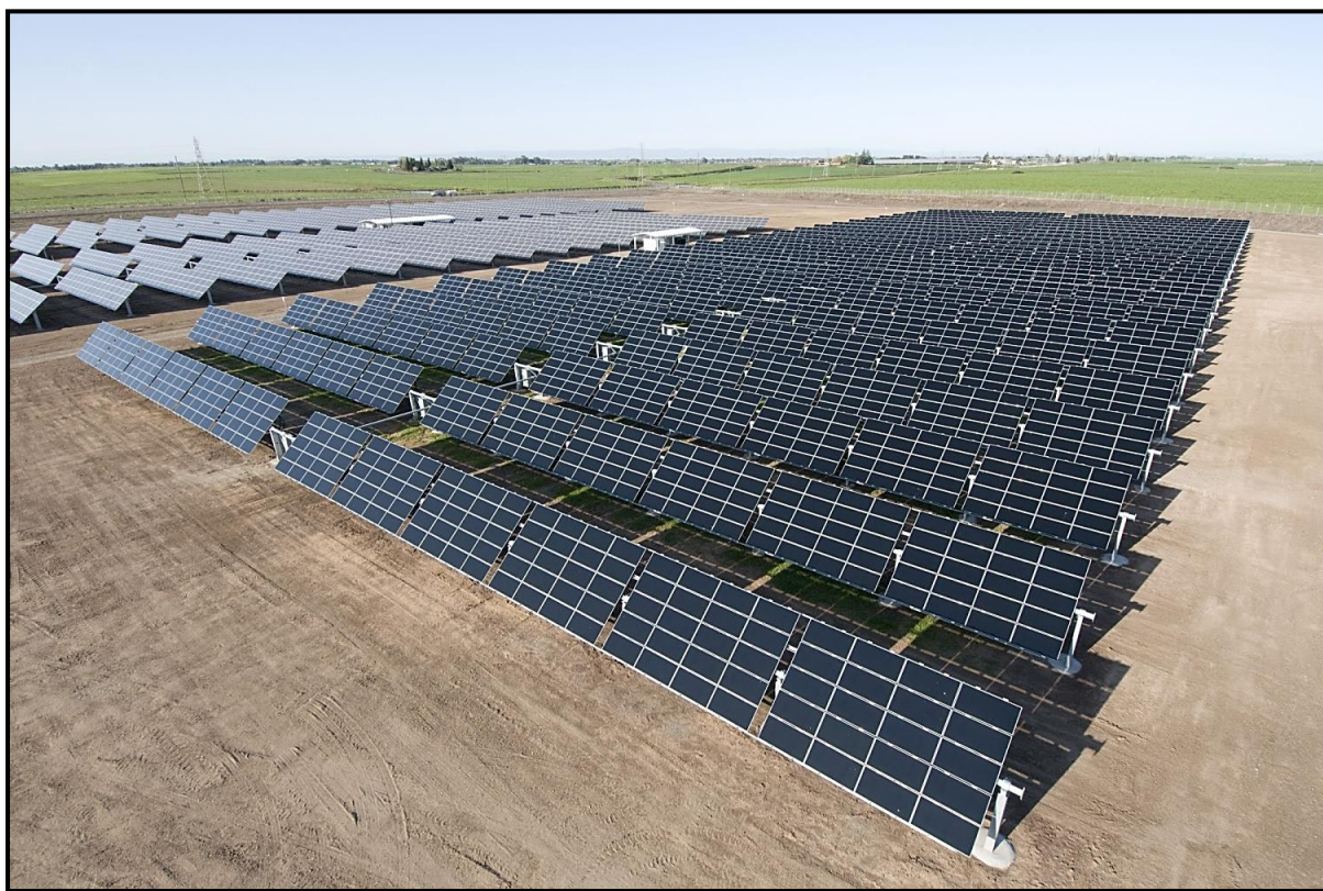
Figure 19: An array of mounted PV Panels
