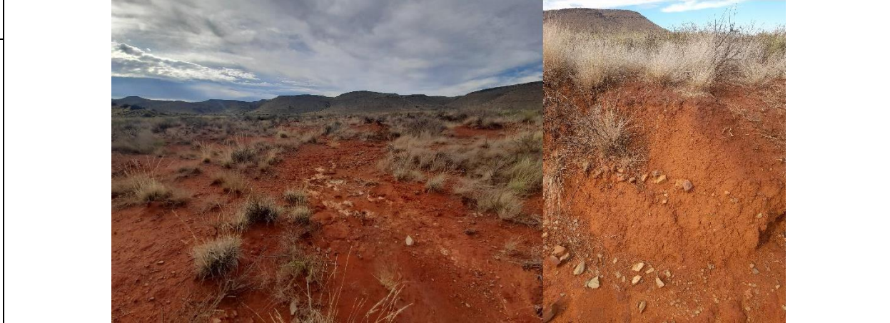
Photograph notes: Top: The narrow channels of two of the EDL's; Bottom left – area where one of the EDL's dissipates; Bottom right – Example of bank erosion along one of the EDLs.
