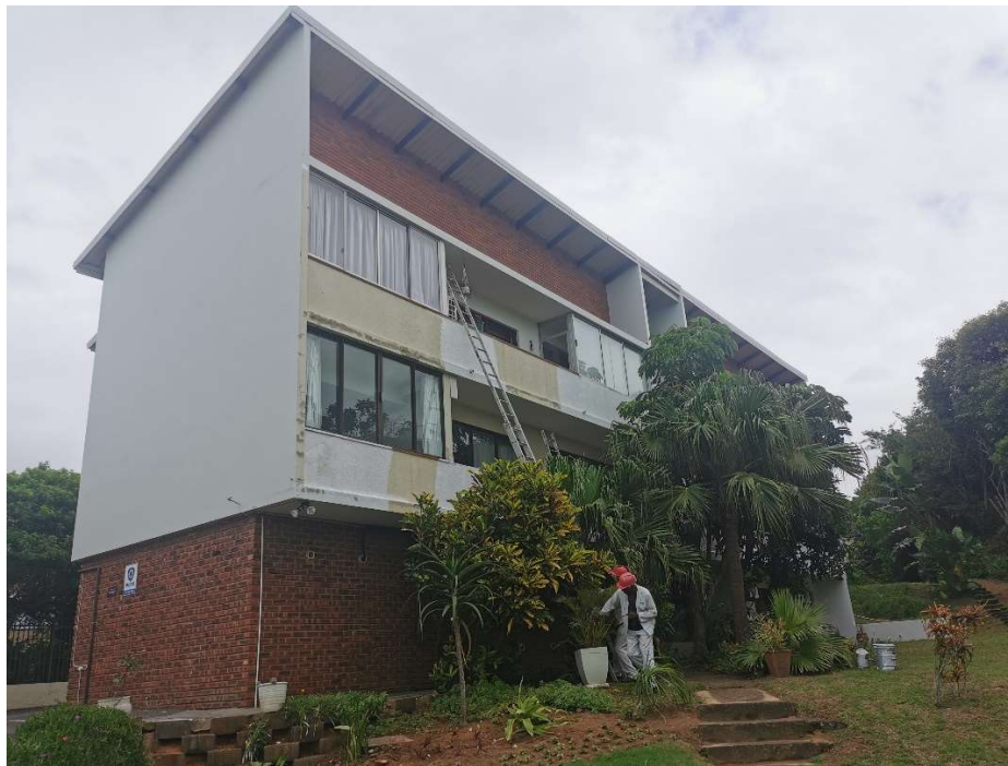
PHOTO 02 – VIEW FROM NORTH EAST – THE EXISTING UNIT 01 (WORK IN THIS PHOTO SHOWS EXTERNAL PAINTING TO THE COMPLEX ONLY)
