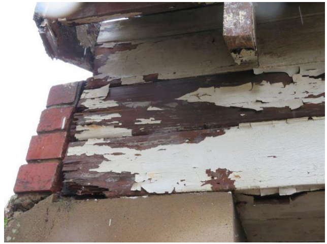
Photo 44: Timber beam showing signs of rotting
