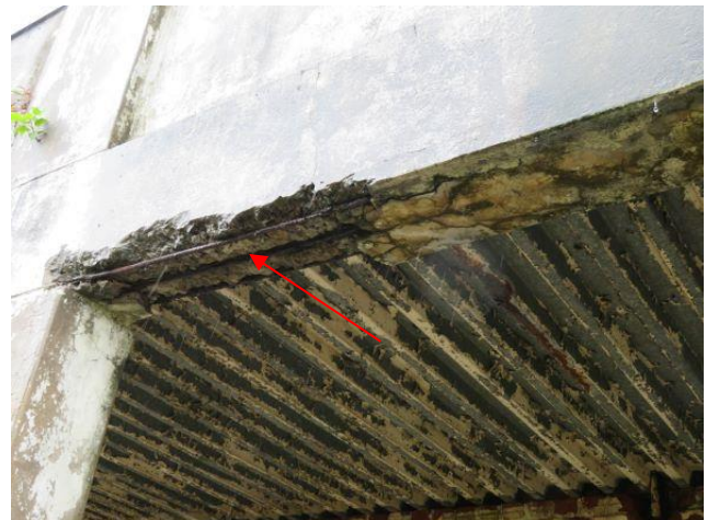
Photo 30: Spalling Concrete & Rusting Composite Slab Steel Deck
