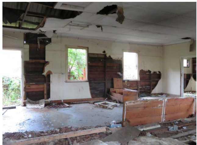
Photo 60: Poor Interior Condition of the Structure
