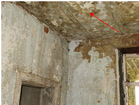
Photo 33: Very Poor Condition of RC Slab Soffit Signs of Cracks and Water Ingress through Slab
