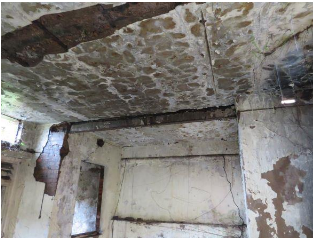
Photo 11: Very Poor Condition of RC Slab Soffit Signs of Water Ingress through RC Slab
