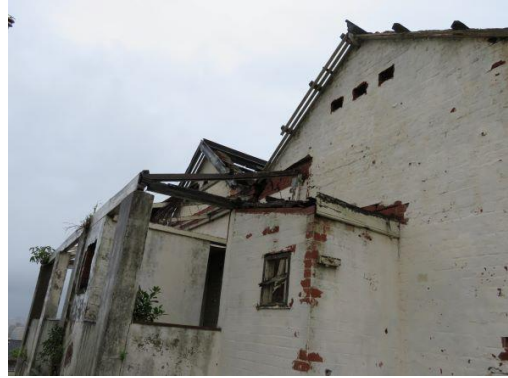
Photo 26: Collapsing Roof Structure
