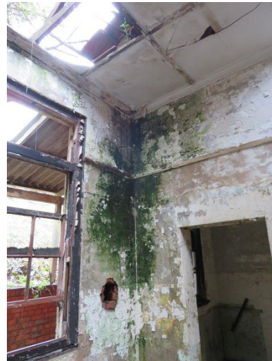
Photo 16: Water damage to walls (noted green mold on walls)
