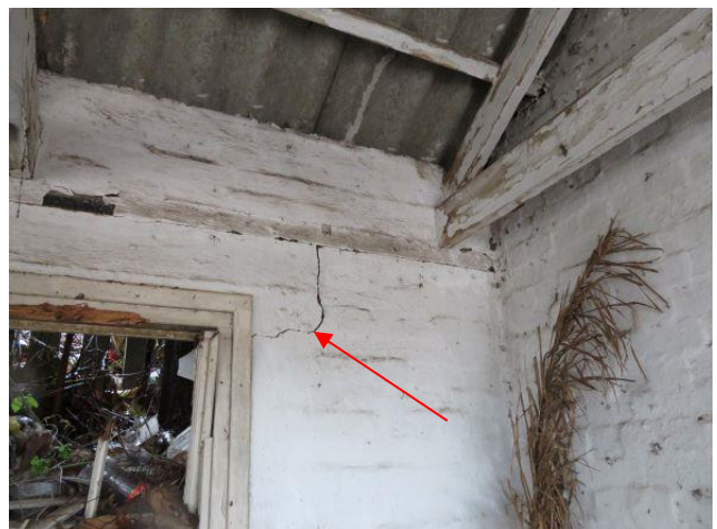
Photo 48: Major cracks on back wall
