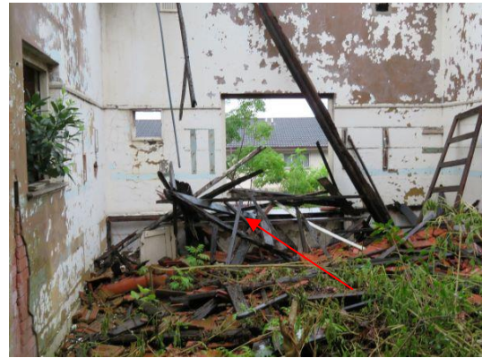
Photo 4: Collapsed Roof Structure Debris
