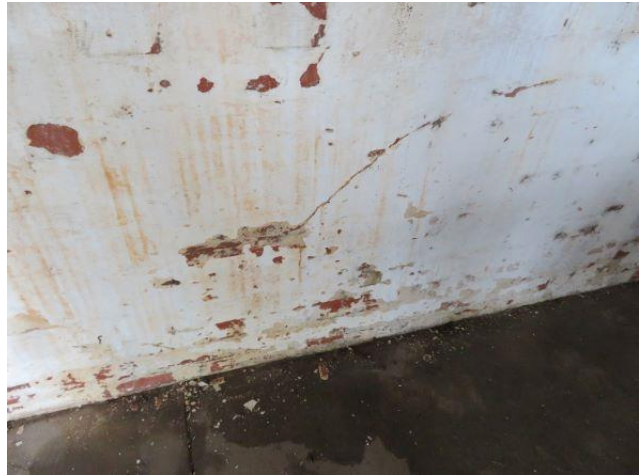
Photo 50: Signs of rising damp on back wall
