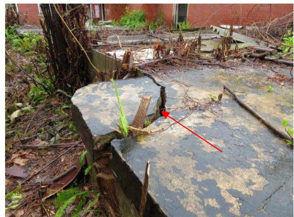
Photo 24: Roof slab showing poor condition (Cracks on slab)
