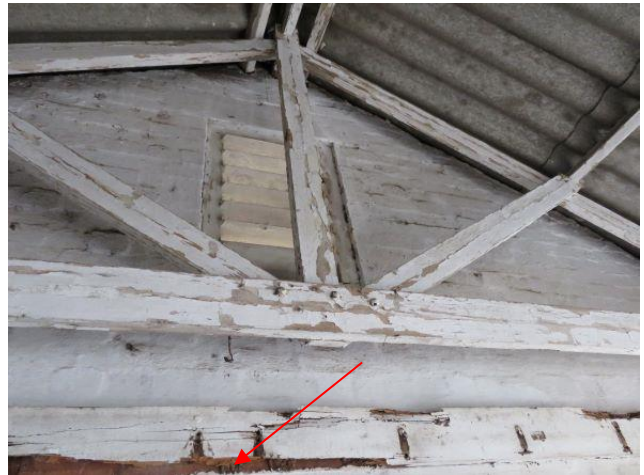
Photo 46: Timber showing signs of rotting
