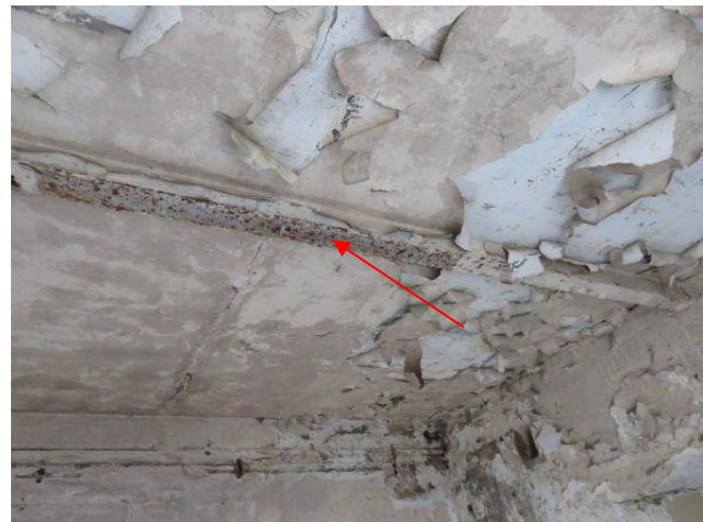
Photo 12: Very Poor Condition of RC Slab Soffit & Rusting Steel Elements
