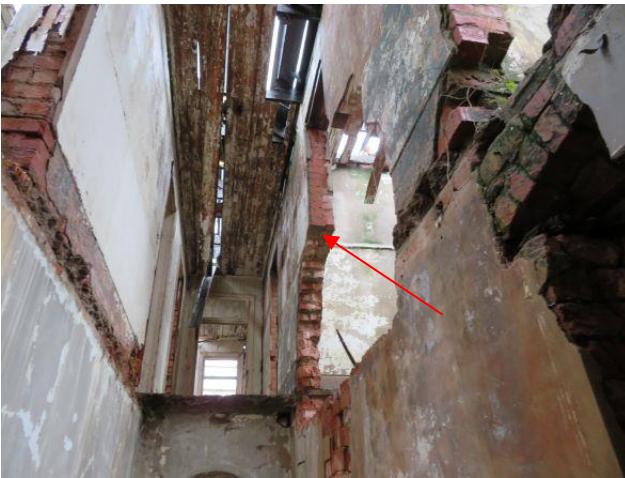
Photo 39: Unsupported Sections of Walls Due to Collapsed / Vandalised Support System
