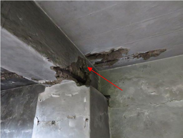
Photo 7: Spalling Concrete and Failure of Beam / Column Connection
