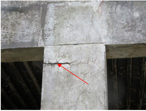
Photo 31: Cracking Beam / Column Connection
