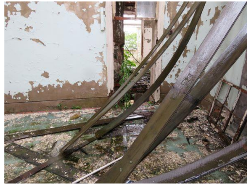
Photo 28: Collapsing Roof Structure Debris
