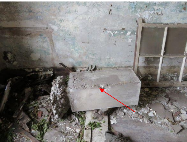
Photo 9: Collapsed RC Element
