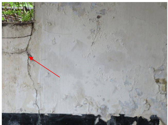
Photo 18: Major Cracks on Walls; Rising damp on walls
