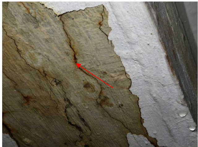
Photo 10: Signs of Water Ingress through RC Slab and Beams
