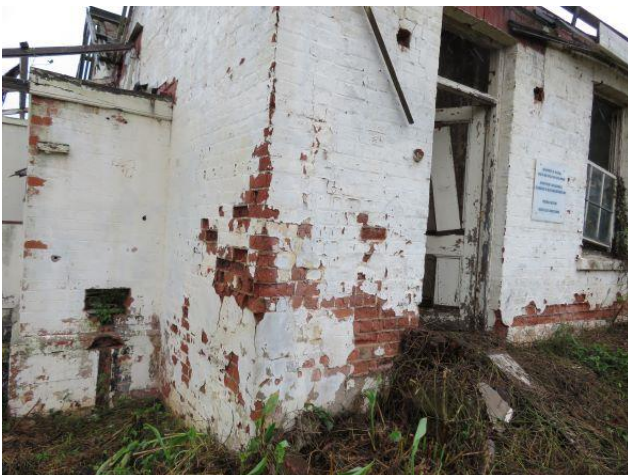
Photo 35: Typical External Wall – Disintegrating Walls and Rising Damp Signs
