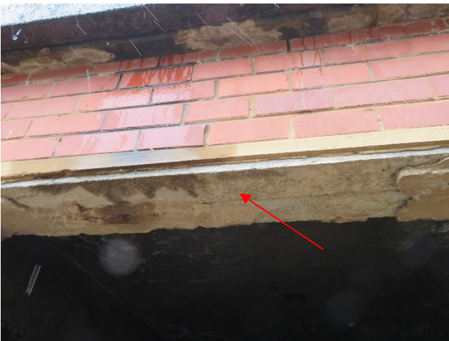
Photo 53: Signs of Lintel Deflection (Plaster delaminating)
