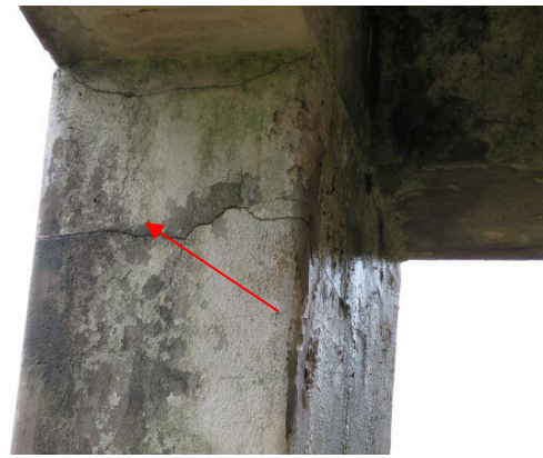
Photo 32: Cracking Beam / Column Connection
