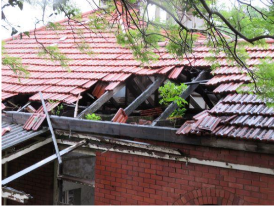
Photo 1: Collapsing Roof Structure
