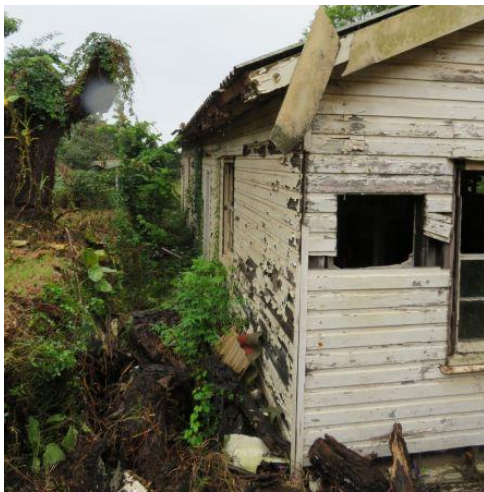
Photo 57: Front View of Building (Note no retaining wall provided)
