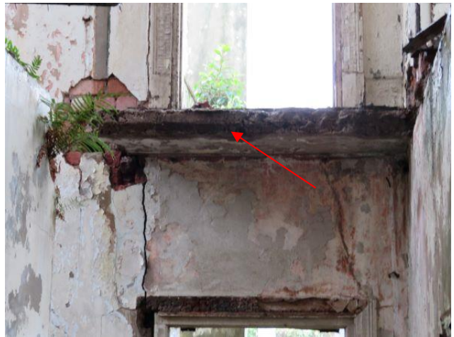
Photo 40: Collapsed walkway slab & Failing lintel system
