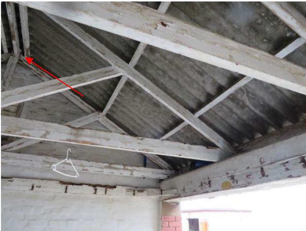
Photo 45: Timber showing signs of rotting
