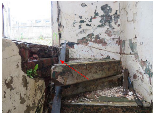
Photo 42: Collapsing Stair Steps (Note poor condition of external wall)
