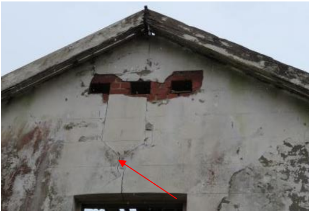
Photo 37: Major Cracks on Gable Wall
