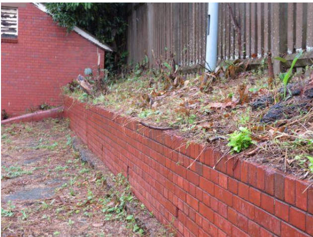
Photo 65: Retaining wall by Main Gate (Note exposed foundations)
