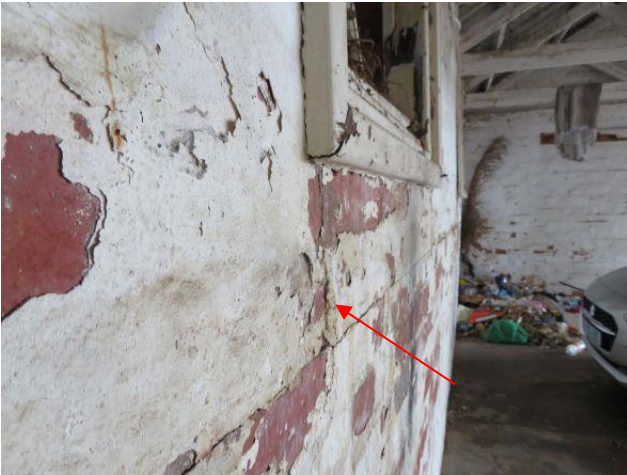
Photo 49: Major cracks on retaining (back) wall (bulging)
