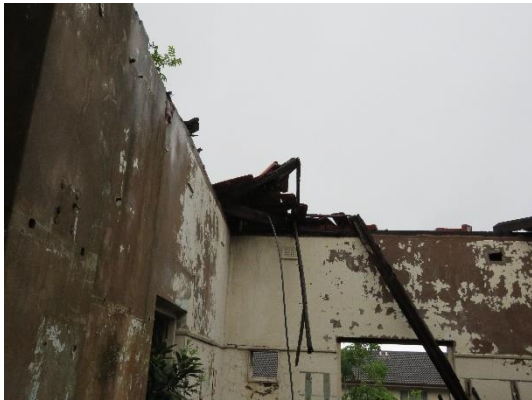
Photo 3: Completely Collapsed Roof Structure
