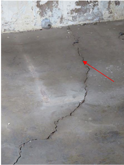
Photo 19: Major Crack on the Surface Bed
