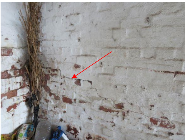
Photo 47: Major cracks on side wall
