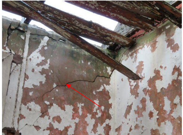
Photo 38: Major Cracks on Internal Wall
