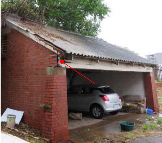
Photo 43: Timber beam showing signs of rotting ( Note asbestos roof sheeting)
