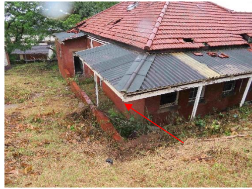
Photo 2: Missing Walkway Roof Corner Timber Column
