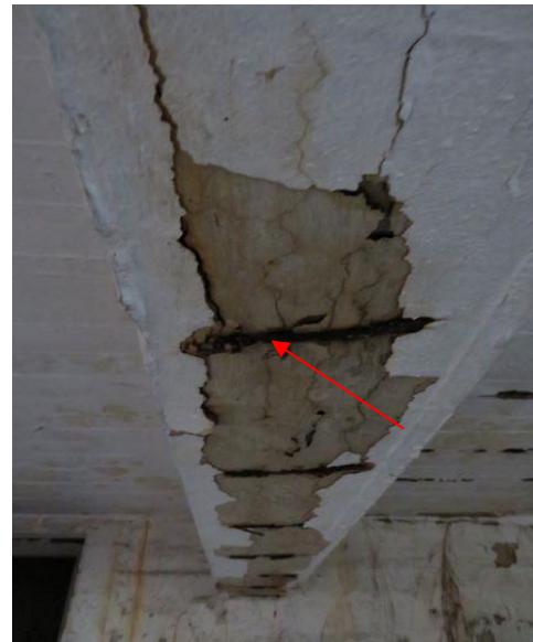
Photo 6: Spalling of Concrete and Rusting Rebar – Basement Roof Beam
