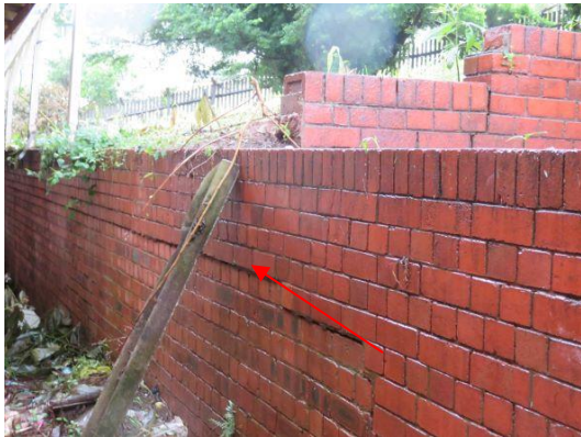
Photo 21: Horizontal Cracks on Brick Retaining Wall
