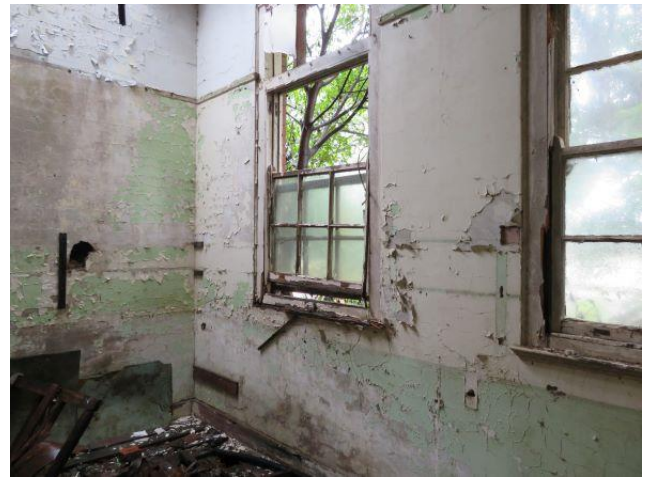
Photo 14: Water damage to walls
