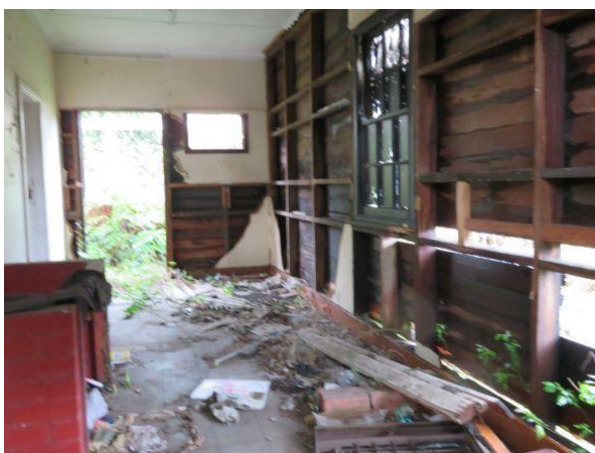
Photo 59: Poor Interior Condition of the Structure
